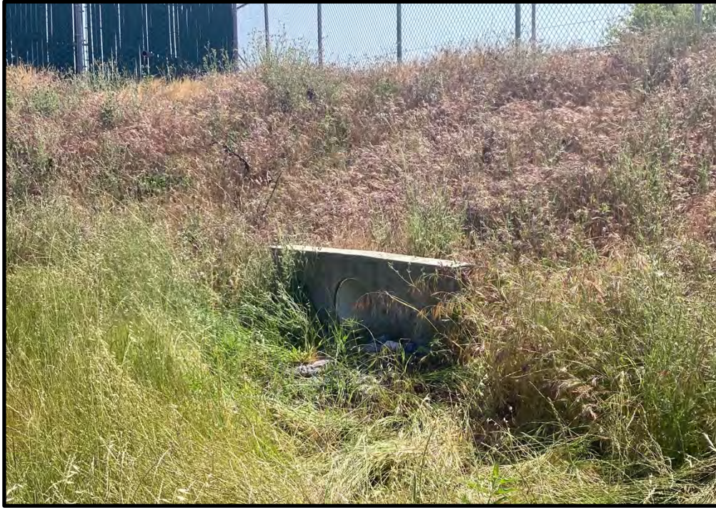
Upstream end of the largest seasonal wetland swale in the site, looking northeast; 05/24/23. Drainage water from the adjacent school is directed into this culvert.
