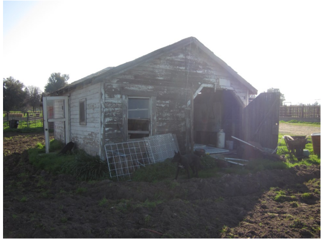
Photo 4: Close up view of the garage. The garage was in a state of disrepair.
