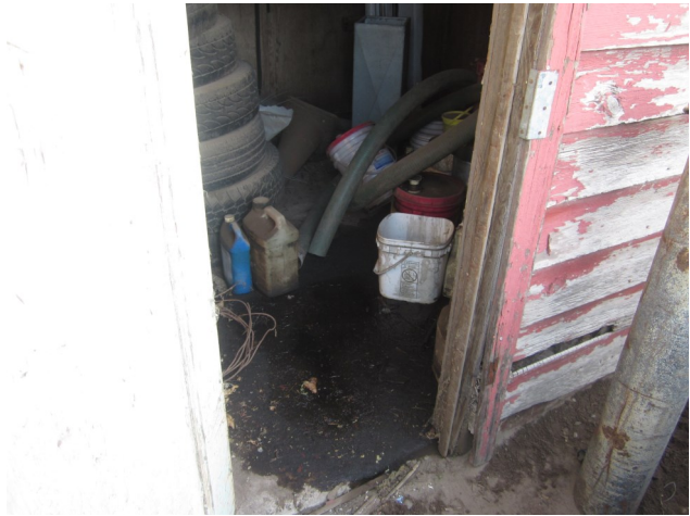
Photo 10: View of the interior of the small shed. A very large oil stain is visible on the floor of the shed.
