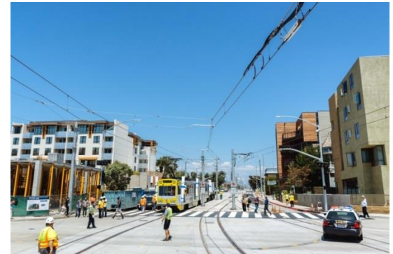
Trained flaggers ensure the safe crossing of pedestrians and workers of an adjacent development.
