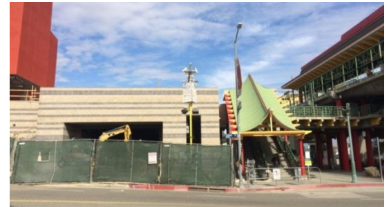
Sidewalk access is blocked for construction project, forcing pedestrians into street or to use less direct paths to the Metro facility.
