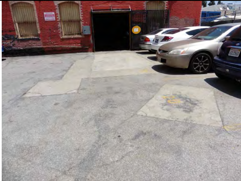
3. Site Exterior: View of several patches noted on the northeast corner of the public parking lot associated with 1240 South Hope Street.
