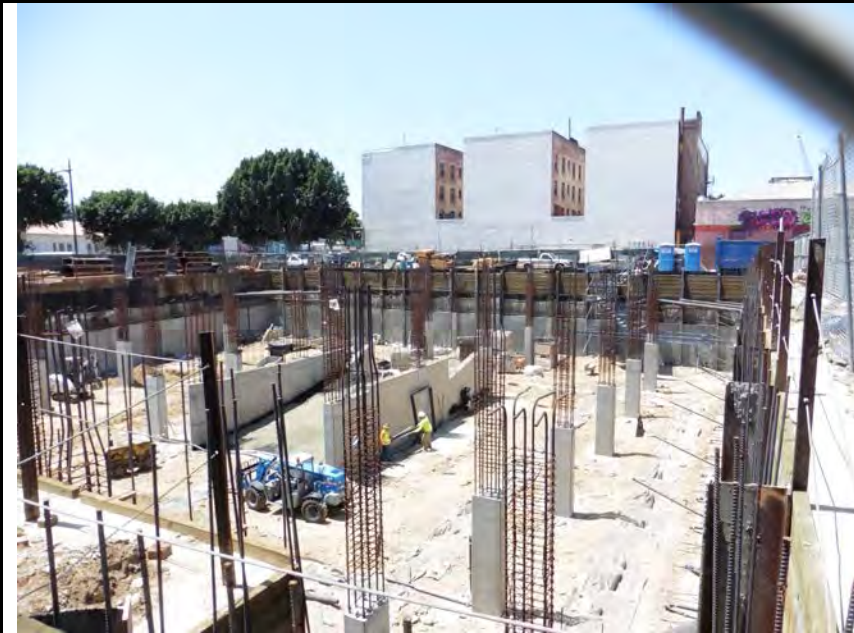
15. Southeast Adjacent: View of a construction site, located on the southern portion of the southeast adjacent property.
