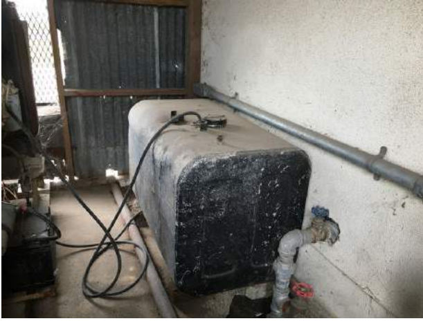
19. View of the 100-gallon diesel AST for the emergency generator located on the subject property.
