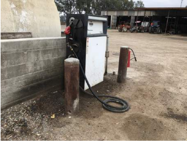
31. View of the fuel pump for the 10,000-gallon diesel AST with staining around the base.
