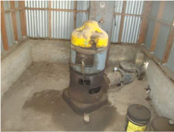
49. View of the interior of an irrigation well pump house with staining noted around the pump.
