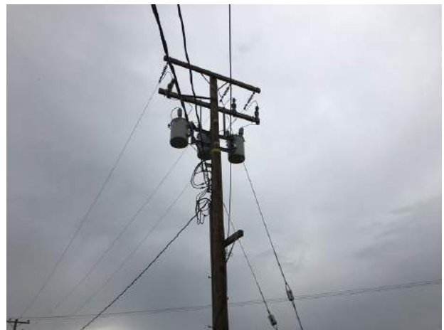
52. View of typical pole-mounted transformers located along the northern portion of the subject property.
