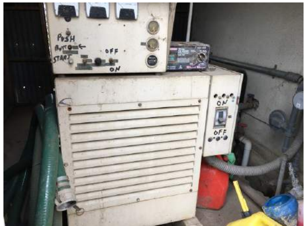
18. View of the emergency generator located near the northwestern portion of the main milk barn of the subject property.
