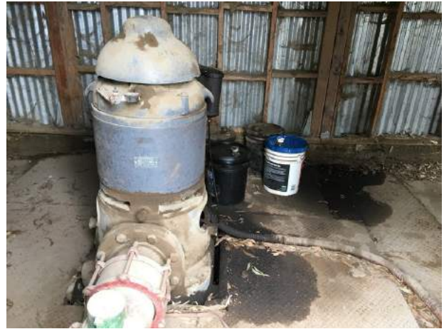
50. View of the interior of the additional irrigation well pump house with staining noted around the pump.
