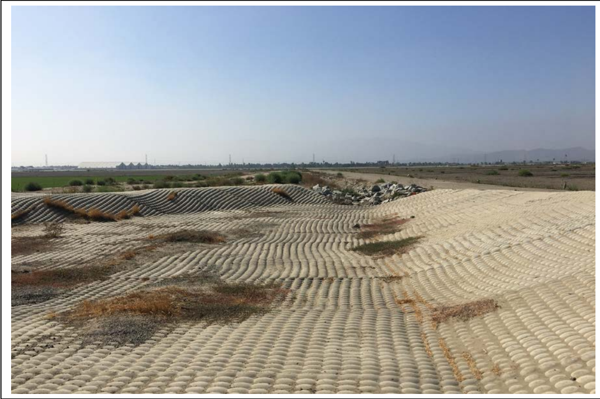
Photograph 9: View to the south of a concrete-lined portion of the Grove Channel, located within a portion of the Chino Airport.
