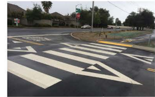
Raised High Visibility Crossing
