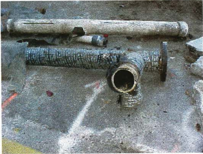
typical product piping (S.W. Steel, corrugated) - no evidence of waste release.
