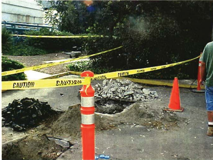
Sample T2-2 at 10000 gallon tank
