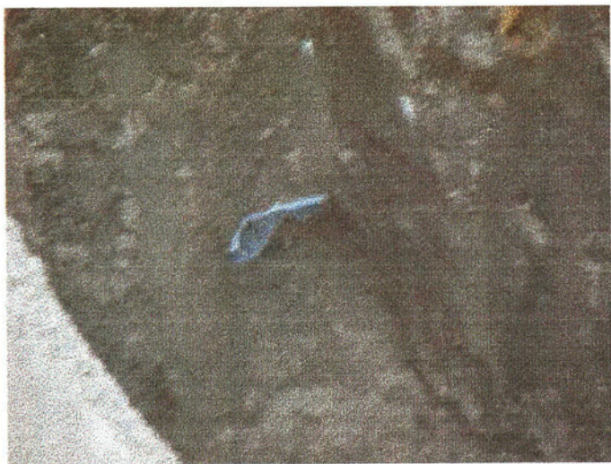
Blue PVC piping in tank exc. to be concrete capped and plugged
