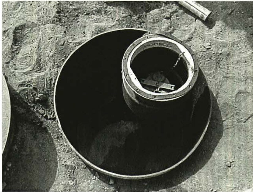
NEW OVERSPILL BUCKET IN FILL SUMP
