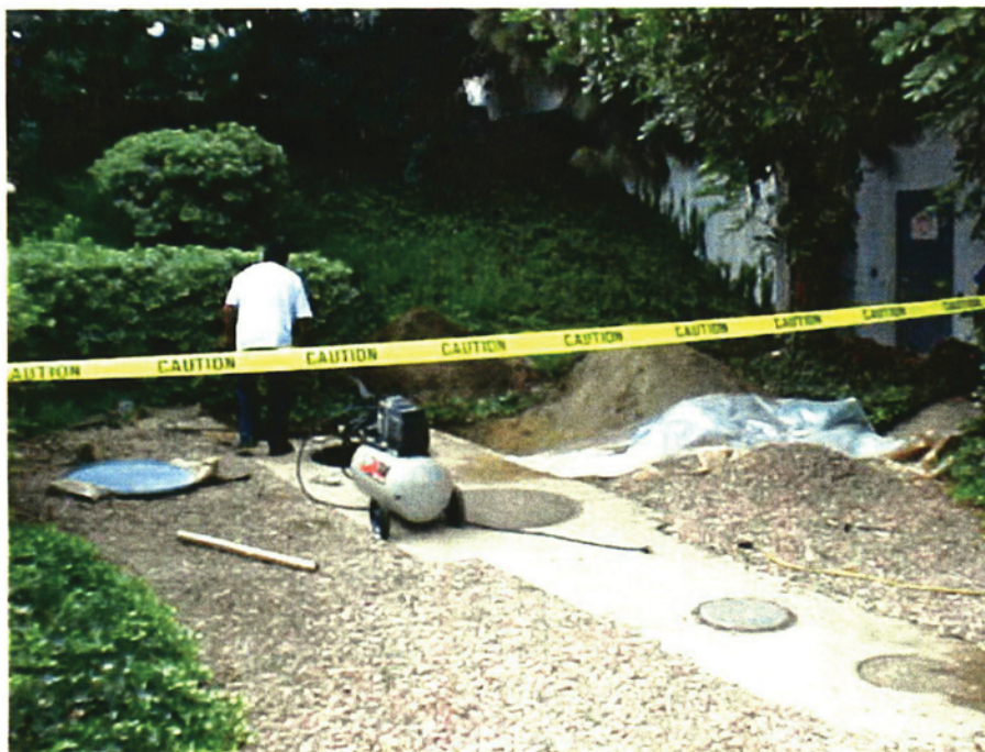
Sample T2-5 at the 10000 gallon tank
