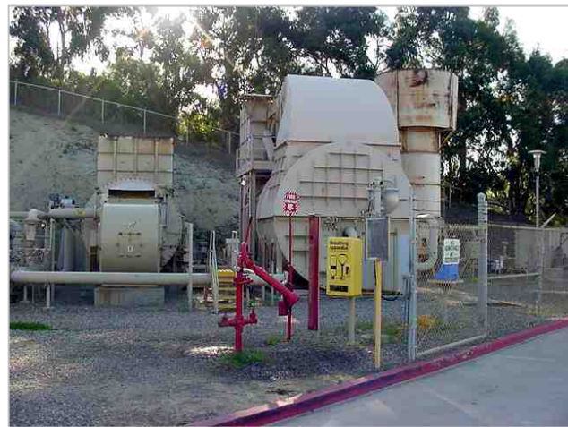
Oil Processing Equipment at the Venoco Ellwood Onshore Oil Gas and Processing Facility
