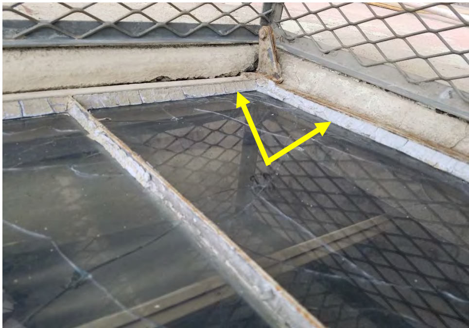
Photograph 2: Building 1: view of asbestos-containing window putty.
