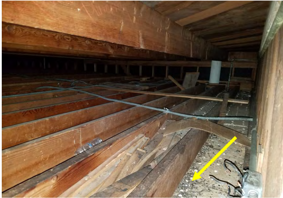
Photograph 15: Shed 1: view of rodent feces throughout ceiling plenum.
