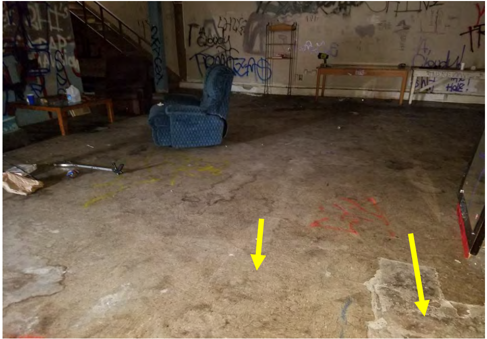
Photograph 5: Building 1: view of asbestos-containing 1'x1' vinyl floor tile and mastic.
