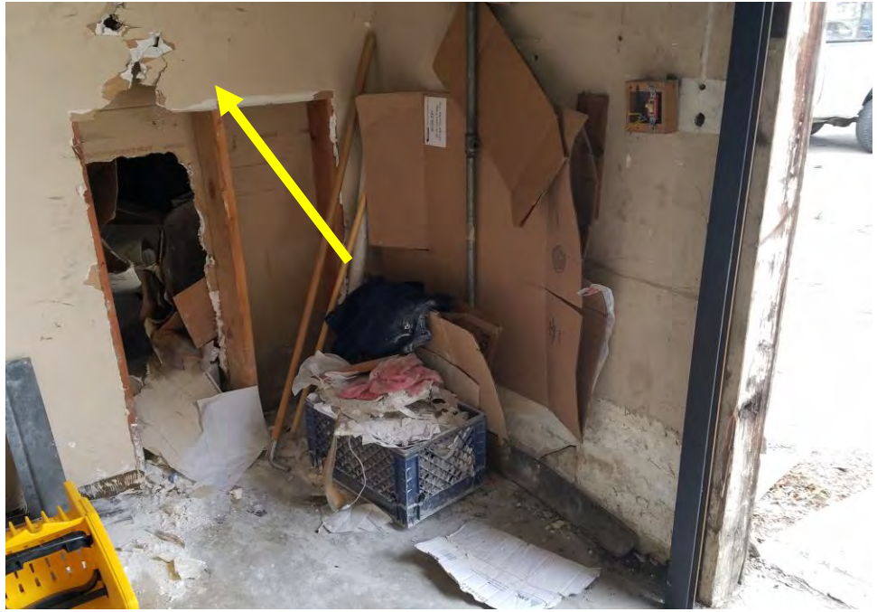
Photograph 11: Building 2: view of asbestos-containing joint compound associated with drywall.
