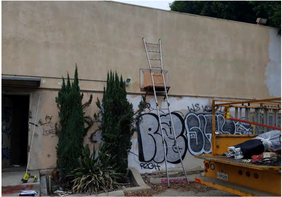
Photograph 3: Building 1: view of asbestos-containing exterior stucco.
