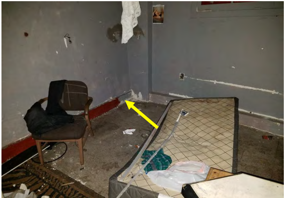
Photograph 4: Building 1: view of asbestos-containing baseboard plaster.
