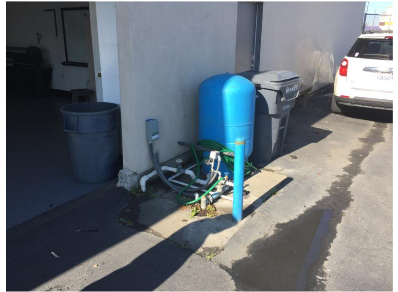
Photo 6: View showing domestic well at 2612 Santa Rosa Avenue
