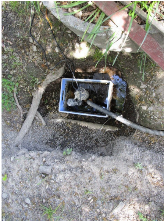
14. Sump pump adjacent to the office
