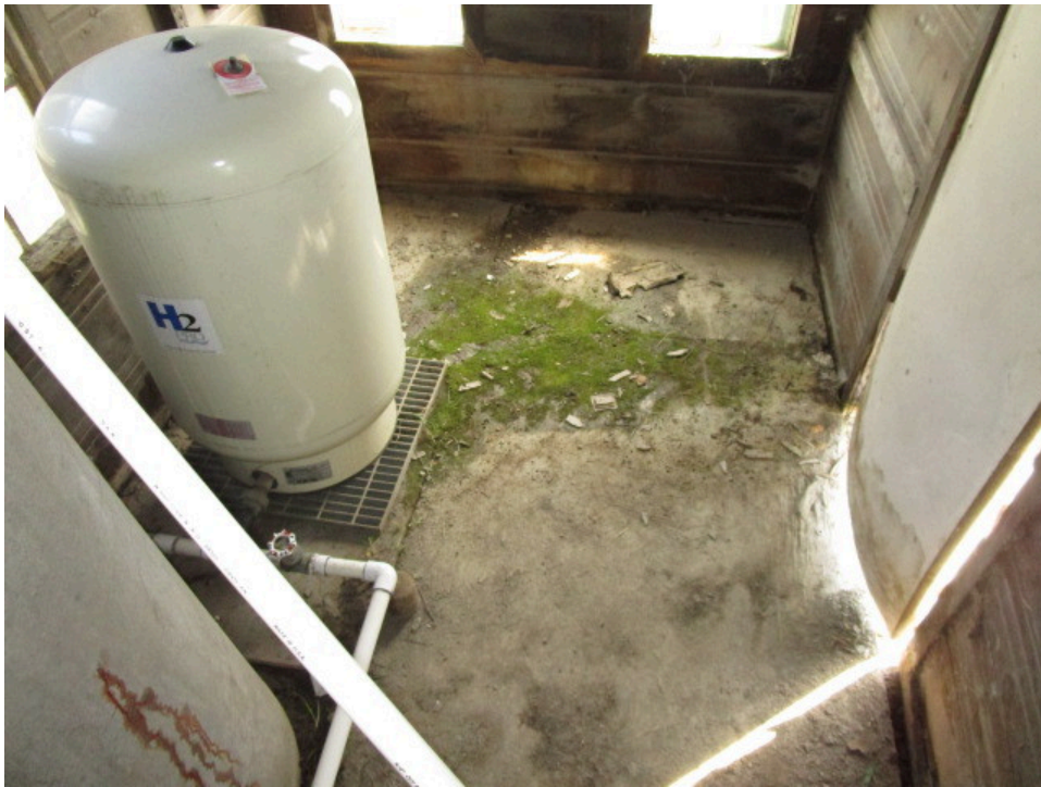
42. Apparent pressure tank in the shed
