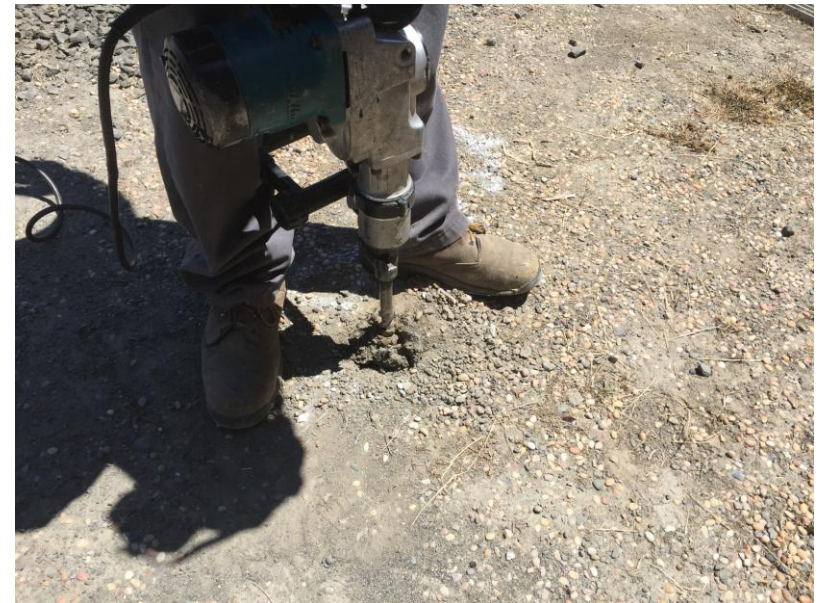
Photo 4: View removing upper 3 feet of hydrated BenSeal prior to completion of soil vapor probe with neat cement
