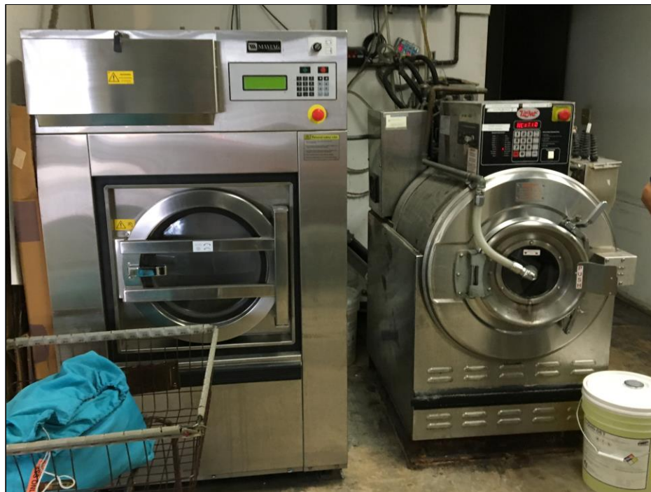
Photograph No. 14 Maytag commercial washing machines inside Clairemont Village Cleaners.
