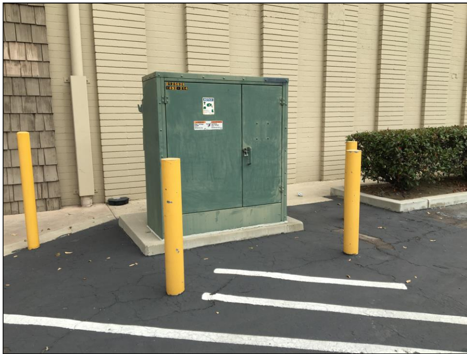
Photograph No. 31 Pad-mounted transformer observed near Rite Aid on the northeastern portion of the Site.
