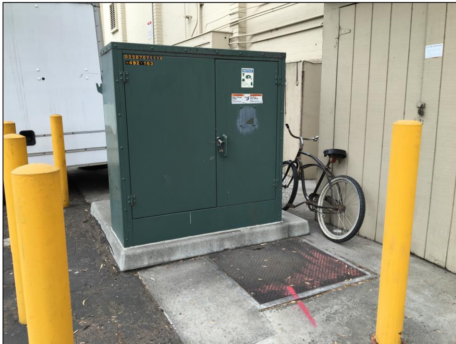
Photograph No. 32 Pad-mounted transformer observed east of Keils on the southeastern portion of the Site.
