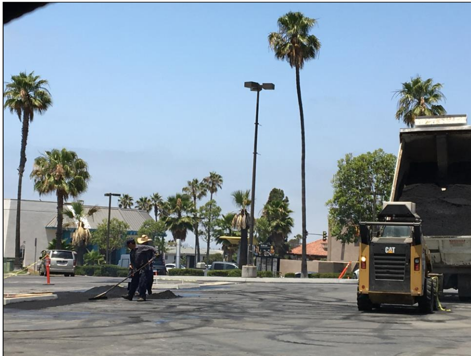
Photograph No. 6 View to the southwest of the parking lot repair process.
