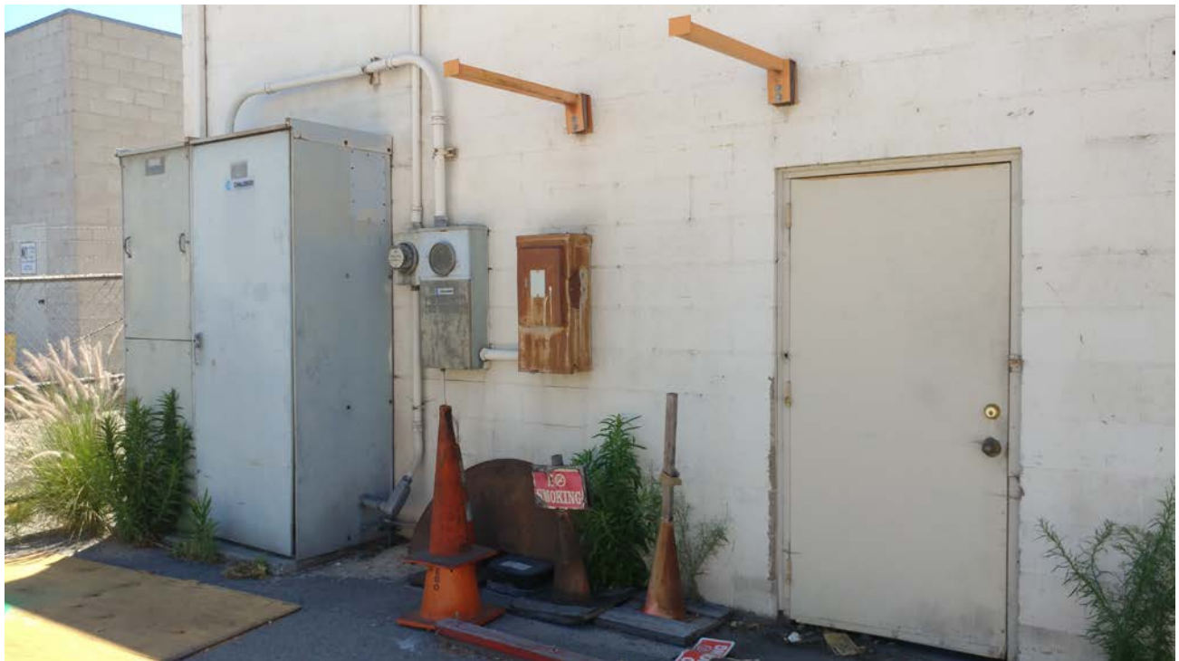
Overview of utility area at northeastern façade of Warehouse B, looking southeast.
