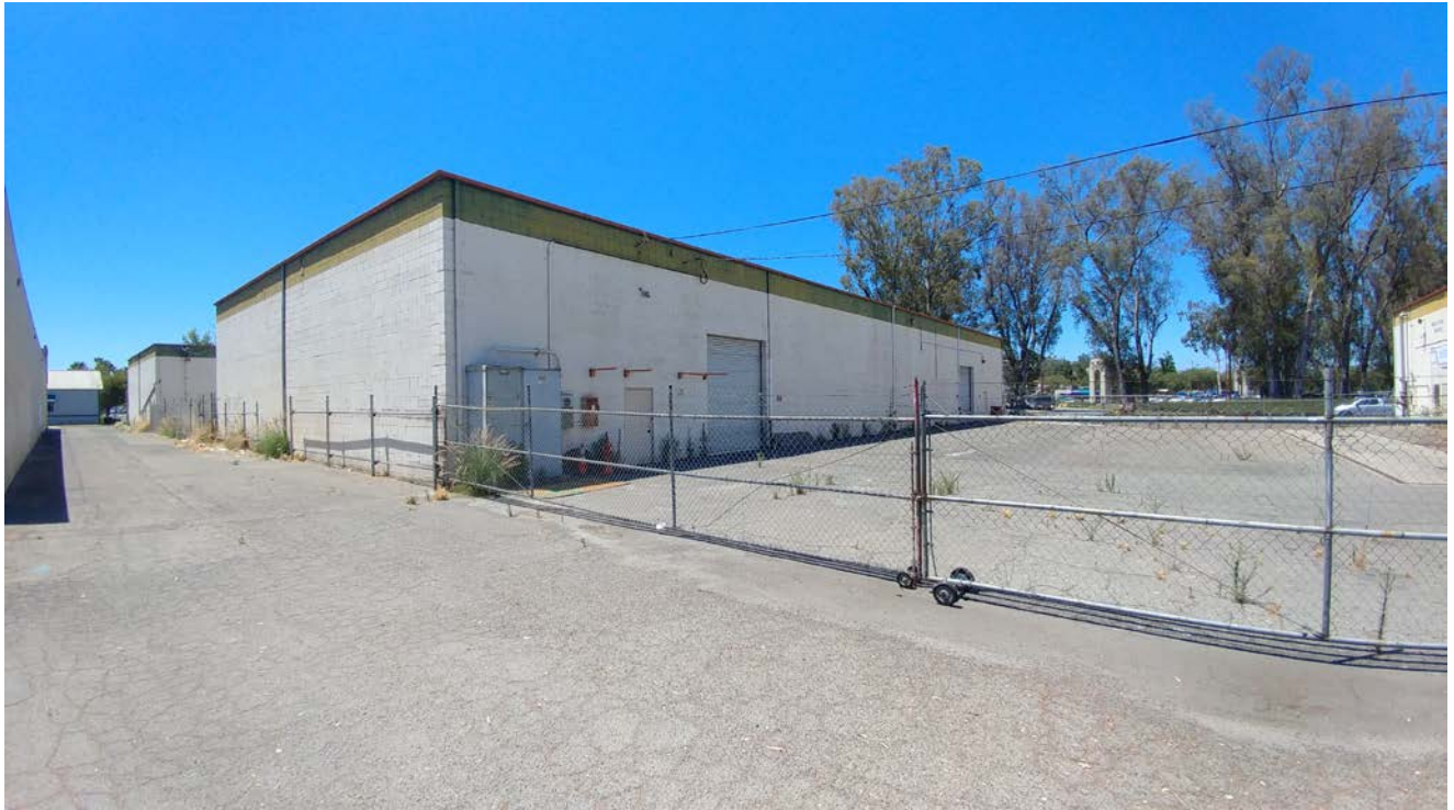
Overview of northern façade of Warehouse B, looking southwest from the alleyway along the east of the property.
