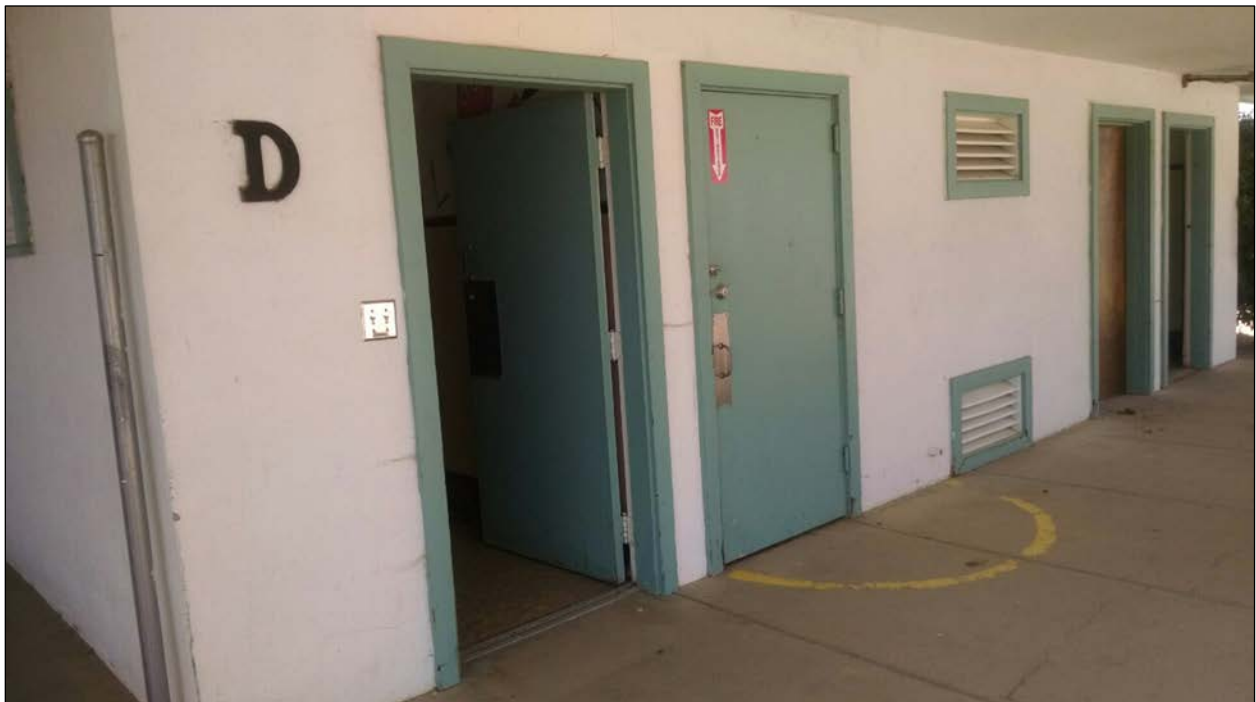
Figure 67. Bathroom entrances (facing main covered walkway), Classroom Building D; girls' bathroom on left, boys' bathroom on right.
