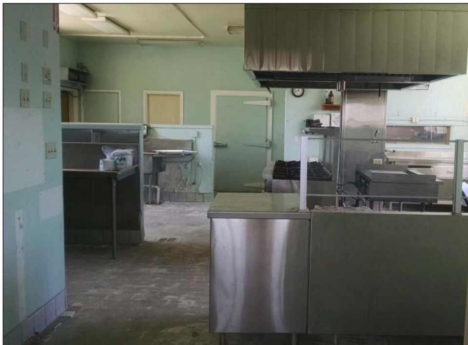
Figure 31. General view of kitchen attached to multi-purpose room. Food storage locker on rear wall; doorway at left leads to storeroom and rear parking lot. Tile flooring partially removed. Stainless steel equipment in place.
