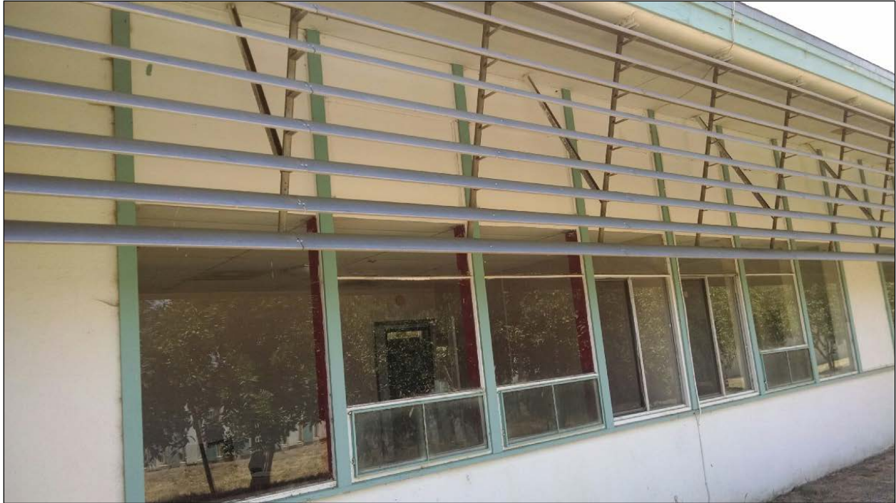
Figure 54. View of expansive window ribbons (with small operable sash elements) and louvered screen system on north elevation of Classroom Building C.
