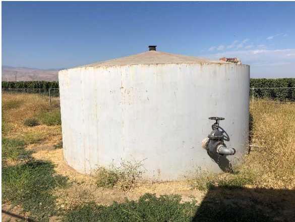
Photo #7 Onsite water tank for fire suppression, facing southeast.
