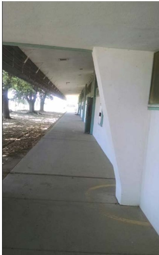
Figure 75. Angled architectural element separating bathrooms from classroom on south side of Classroom Building D.
