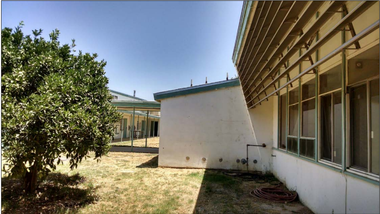
Figure 53. View east along north wall of Classroom Building C and attached bathroom, toward Building A corridor.
