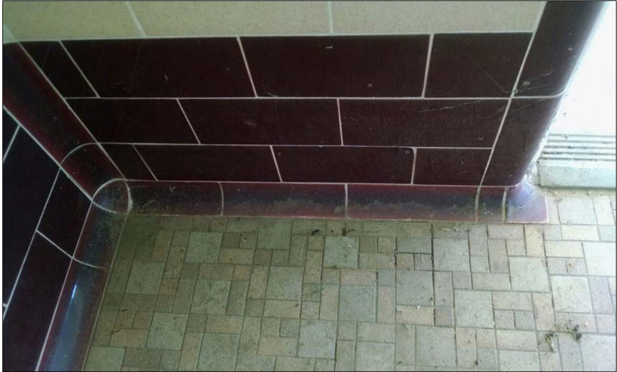
Figure 66. Ceramic wall tile in boys' bathroom; floor tile is probably a replacement.
