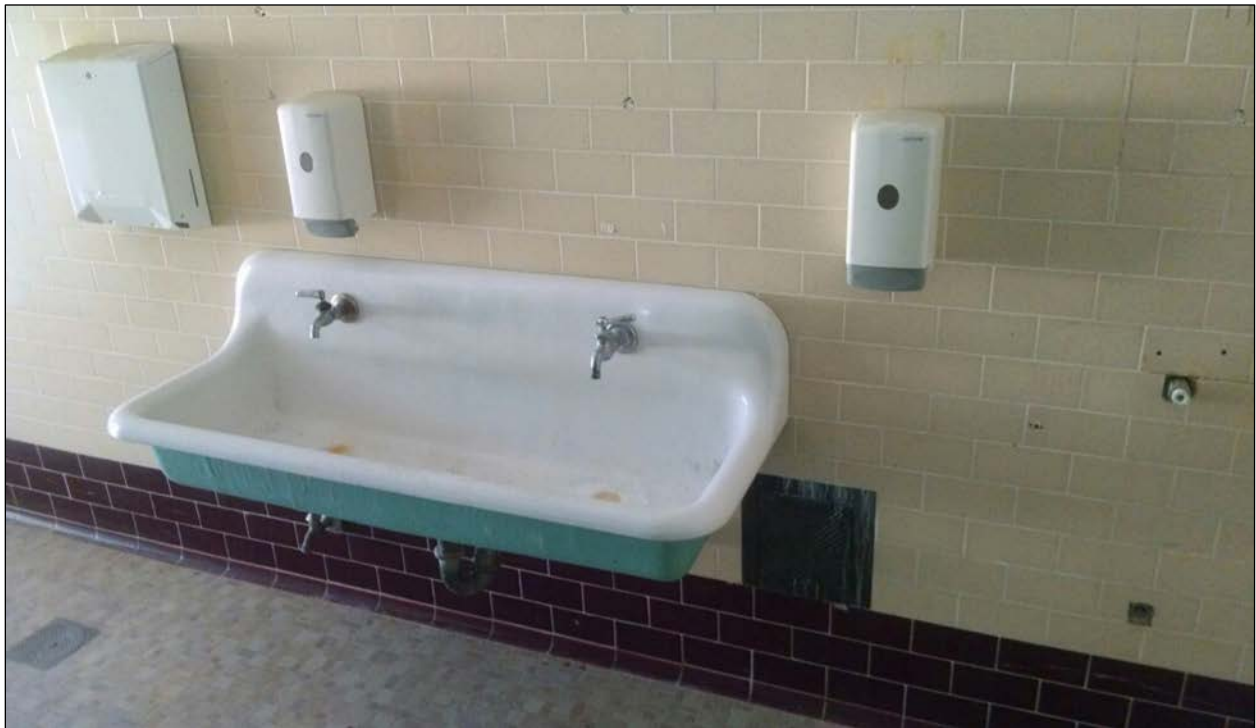
Figure 69. Original ceramic wall tile in girls' bathroom, Classroom Building D.
