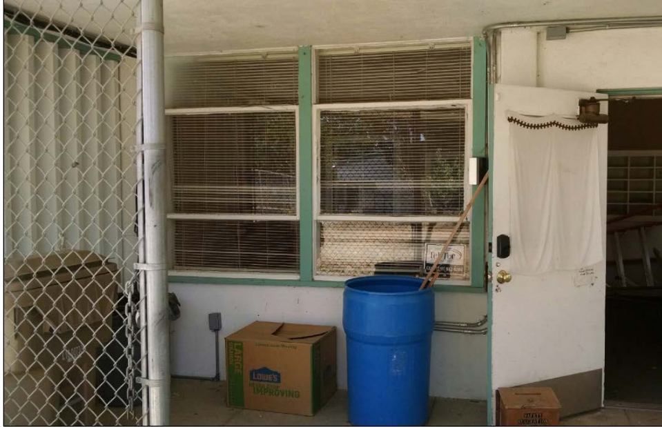
Figure 16. Entrance to administrative office in Building A. Paired vertical tripartite windows in front wall (with operable hopper windows as the center sash); note lack of window frame at upper edge—a standard design feature throughout the campus. Vertical wooden (fixed) louvered screen on left, behind chain-link gate.
