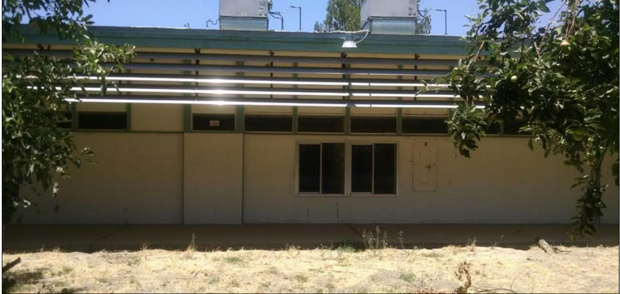
Figure 56. View toward the north elevation of the western portion of Classroom Building C; note the replacement windows.
