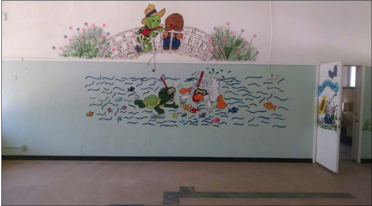
Figure 70. Classroom Building D interior, with original flooring; doorway at right leads to girls' bathroom. Decorative wall painting not original.
