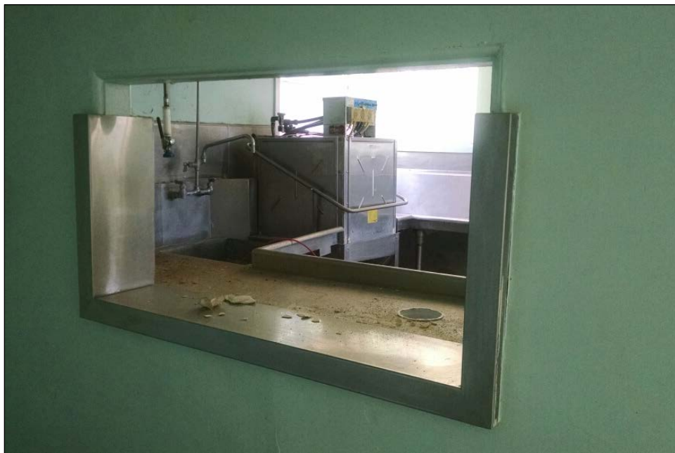
Figure 33. Kitchen tray return. Stainless steel equipment in place.
