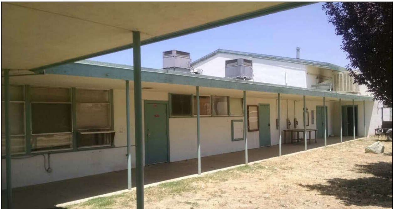
Figure 21. View along corridor from administrative office toward multi-purpose room; note higher gabled roofline of multi-purpose room
