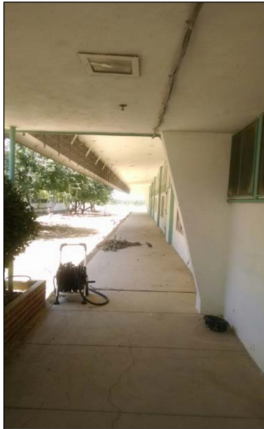
Figure 57. View along corridor on south side of Classroom Building C; note simple, angled architectural element separating classroom portion from bathrooms.
