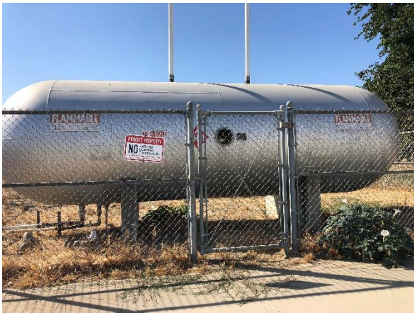
Photo #9 Onsite propane tank, facing south.
