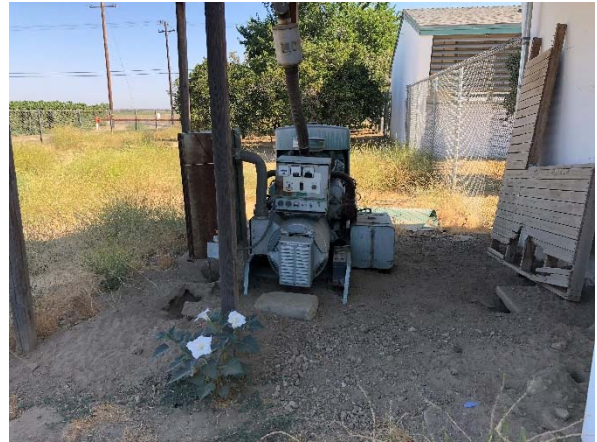
Photo #8 Onsite diesel back-up generator (non-operational), facing north.
