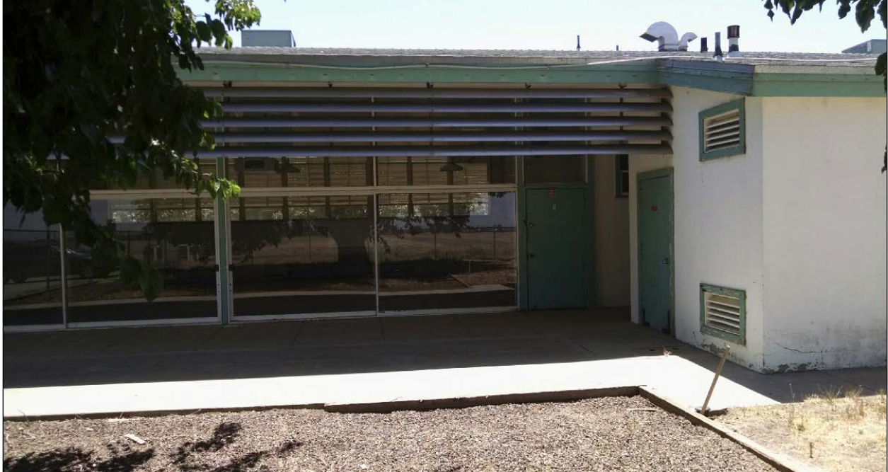
Figure 40. North elevation of Kindergarten Building B, showing exterior of utility room and suspended louvers.
