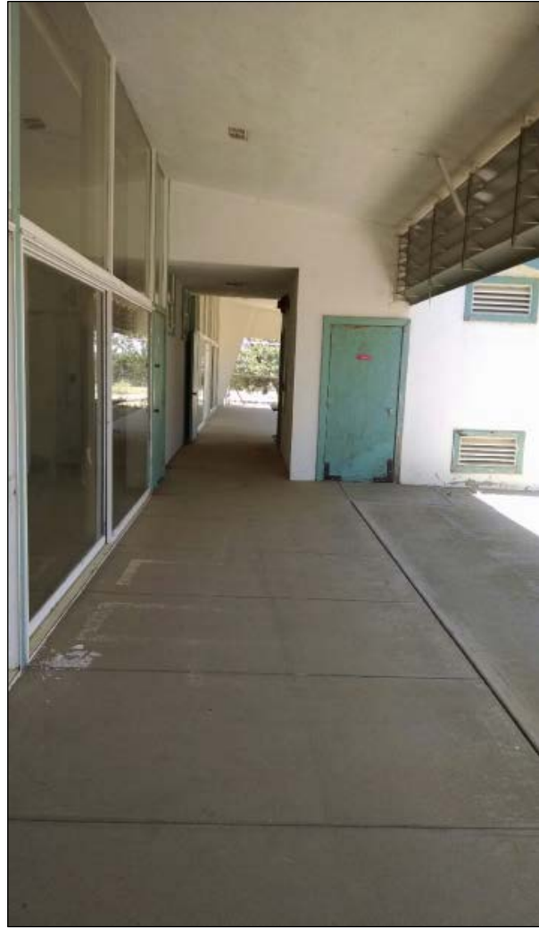
Figure 39. Center of gabled Kindergarten Building B features small utility room with fixed louvered wall vents. Horizontal louvered shades, suspended from outer edge of corridor roof, filter classroom and corridor light.
