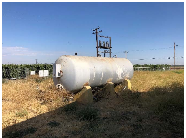
Photo #6 Onsite water storage tank (foreground) and off-site pole-mounted transformers (background), facing west.
