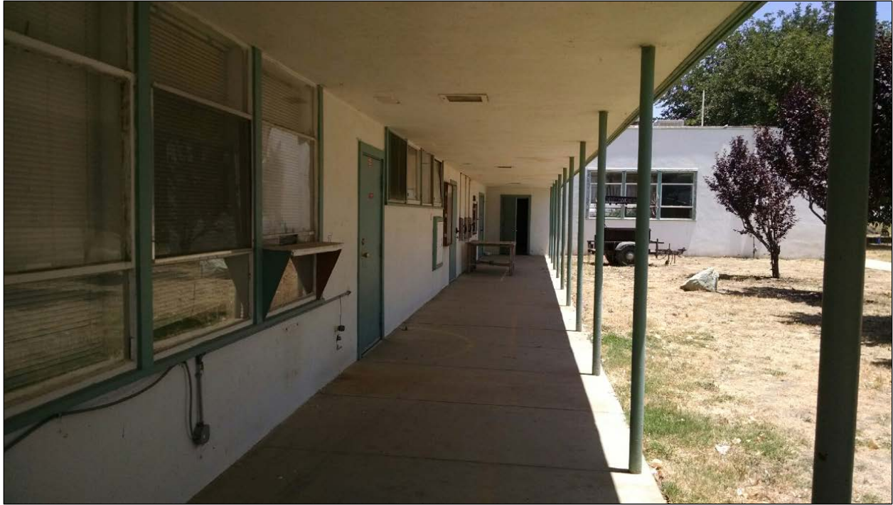
Figure 18. View down covered corridor on south side of Building A, toward kitchen annex and multi-purpose room. Corridor roof canopy supported on steel poles. Corridor ceiling has flush-mounted light fixtures. Original windows (one partly modified with shelf) and doors in place.
