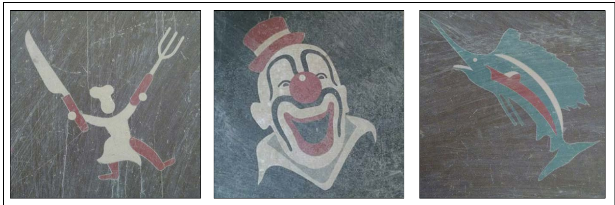
Figure 45. Three Kentile brand "KenSerts" vinyl-asbestos decorative floor tiles (9 x 9 inches) installed randomly in Kindergarten classroom flooring.
