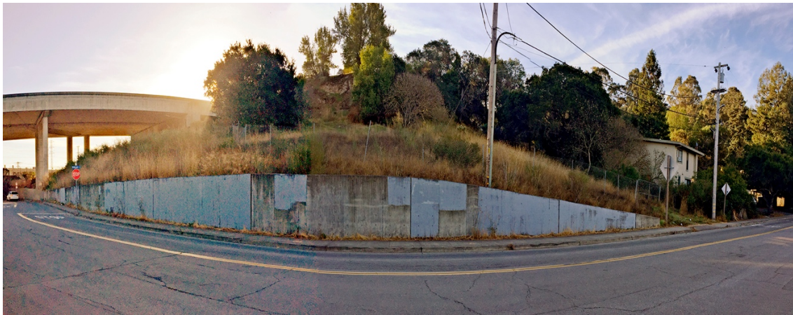
Photo 2. Panoramic View of Lower Portion of the Project Site showing rock face
