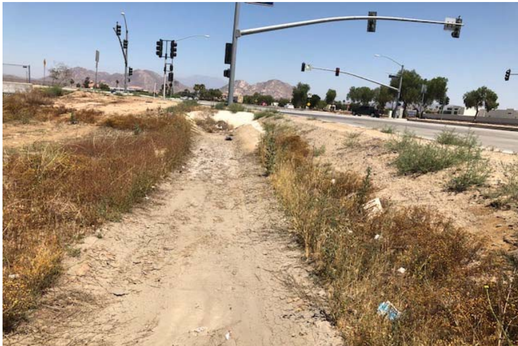
Photograph 5: Easterly view of onsite-ditch with sediment covering the concrete. This photograph was taken at the intersection of Indian Avenue and Ramona Expressway at the southeastern Project boundary.
