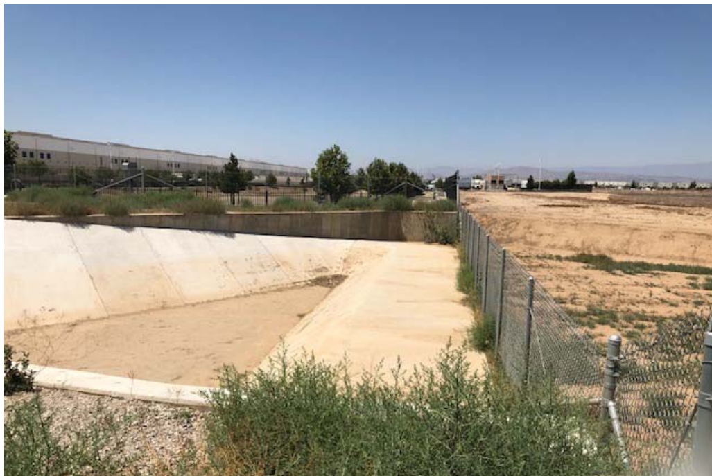
Photograph 4: Easterly view of concrete flood control channel at off-site location where it enters a down-drain and does not flow onto the Project site. Note the lack of a culvert or pipe allowing flow to enter the Project site.
