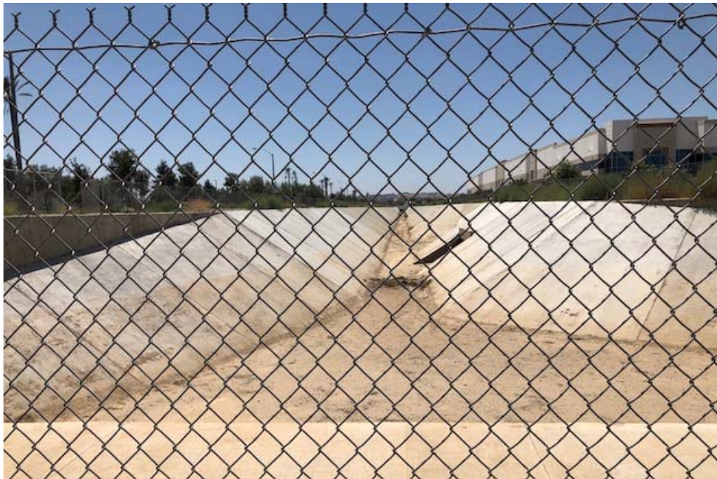
Photograph 3: Westerly view of off-site flood control channel at western Project boundary. Note the concrete sides and bottom for this feature and the down-drain carrying flows underground before entering the site.
