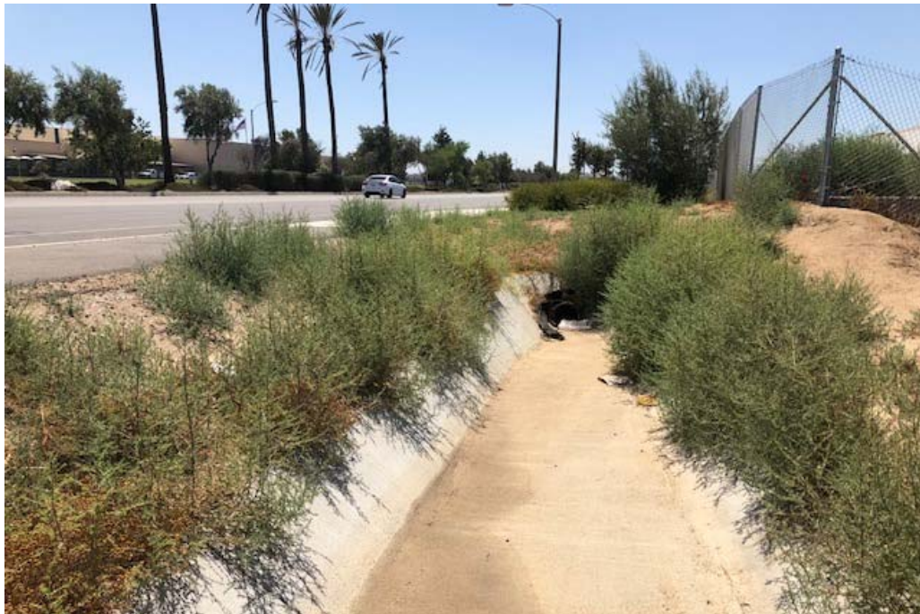
Photograph 1: Westerly view of on-site ditch at Project property boundary. Note the concrete sides and bottom for this roadside ditch.
