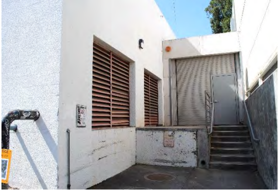
Figure 122. Two large vented openings at the north end of the west façade of Shaklee Building (left), looking south. A hyphen addition attaches to Barclay Simpson Sculpture Studio (right).
