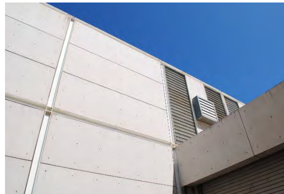
Figure 142. Steel grid structure with fiber-reinforced concrete boards fastened by screws on the east façade, looking west. Metal vents are visible above the central hyphen volume.
