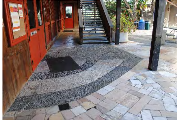
Figure 65. Irregular, polychromatic flagstone and pebble patio between Martinez Hall and Founders Hall, looking south.
