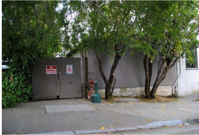
Figure 41. Non-original shed roof addition which abuts the east façade of the Facilities Building, visible at the primary (north) façade, looking south.
