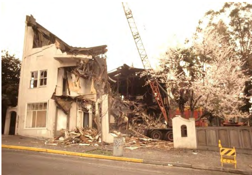
Figure 217. Demolition of Guild Hall after fire in 1971. Source: CCA Libraries Special Collections.
