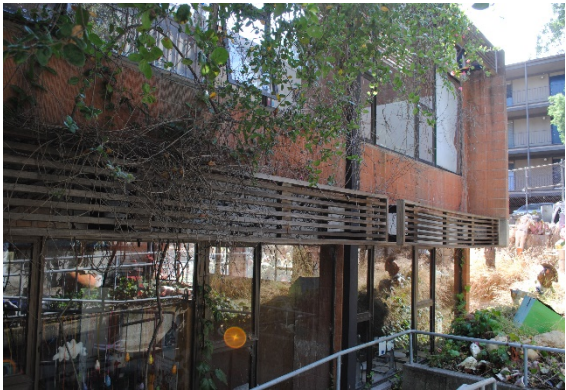
Figure 22. Ceramic Arts Center, portion of south façade with trellis detail, looking northeast
