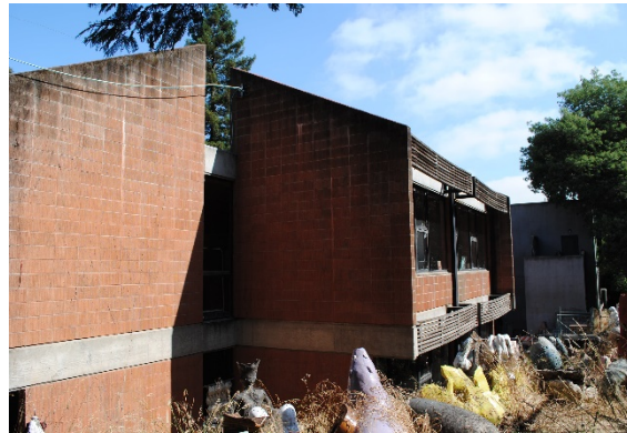
Figure 23. Projecting shed roof volume at the south end of the rear façade, looking northwest
