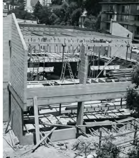
Figure 112. Site clearing and construction of the Noni Eccles Treadwell Ceramic Arts Center, 1973. Source: CCA Libraries Special Collections.
