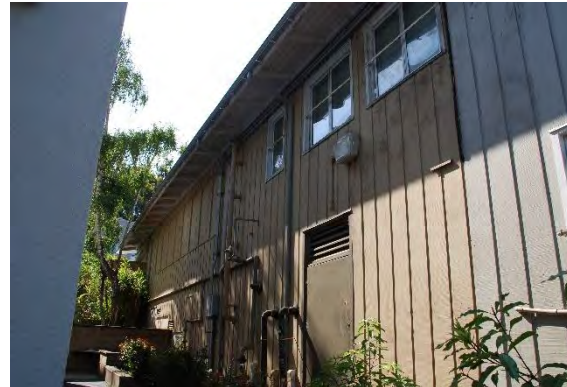
Figure 55. Partial view of the east end of the north façade of Irwin Student Center, looking southeast.
