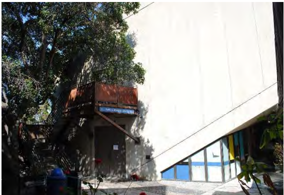
Figure 82. Concrete and metal staircase accessing Nahl Hall within the Founders Hall Building on the east façade, looking south west.
