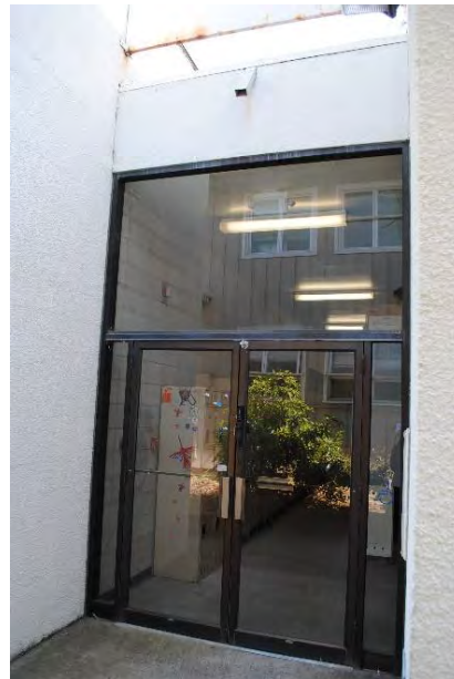
Figure 125. Aluminum storefront window wall with double doors on the south façade of the Shaklee Building, looking north.
