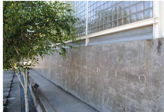
Figure 139. Galvanized metal louvers above the concrete base, within the steel grid frame, looking northeast.
