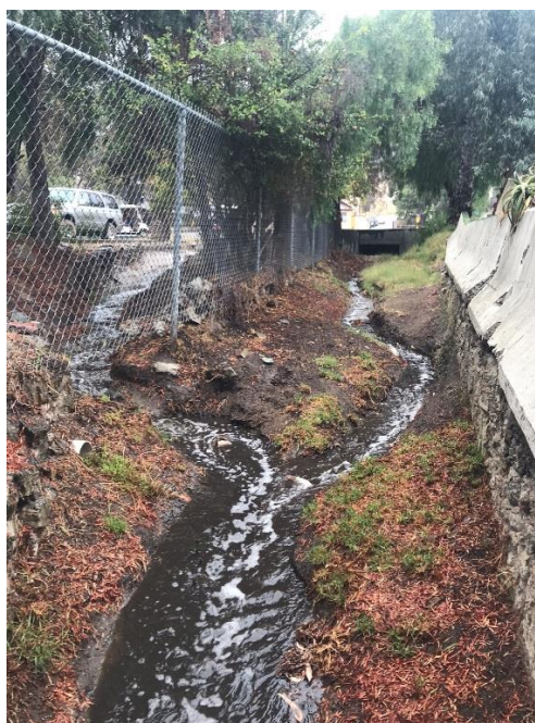
Photo Figure 11: Characteristic conditions of stormwater channel system, in the proposed project area, taken during a rain event at the confluence of the inputs from areas shown in Photo Figures 9 and 10.
