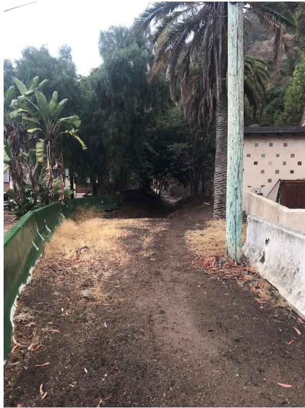
Photo Figure 13: Characteristic conditions of stormwater channel system, in the proposed project area, taken during a rain event below areas shown in Photo Figures 12, 11, 10, and 9.
