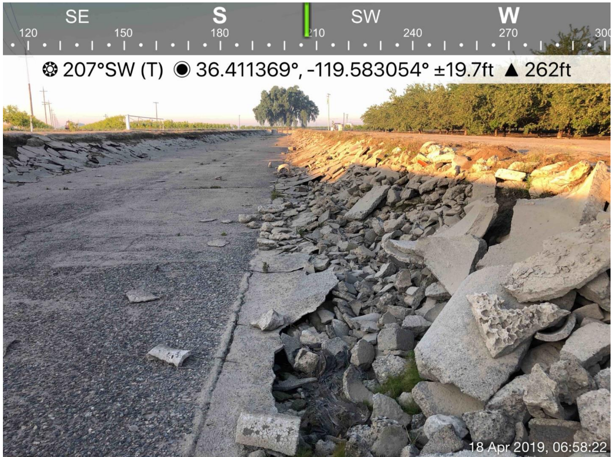
Photograph 2: Lined portion of the channel of People’s Ditch. Rip-rap is present along the banks.
