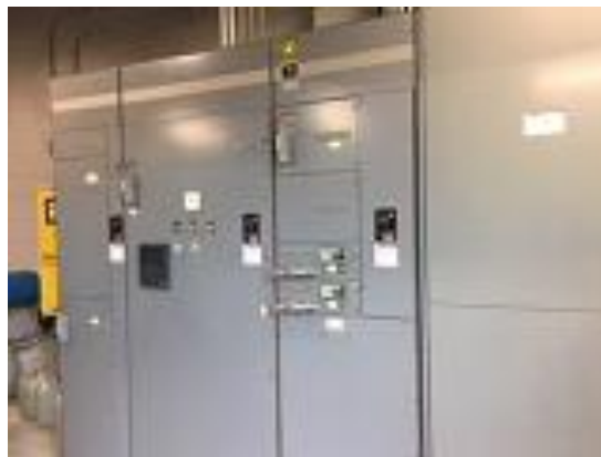
Figure 6.1. Existing SES/RVAT/MCC lineup
