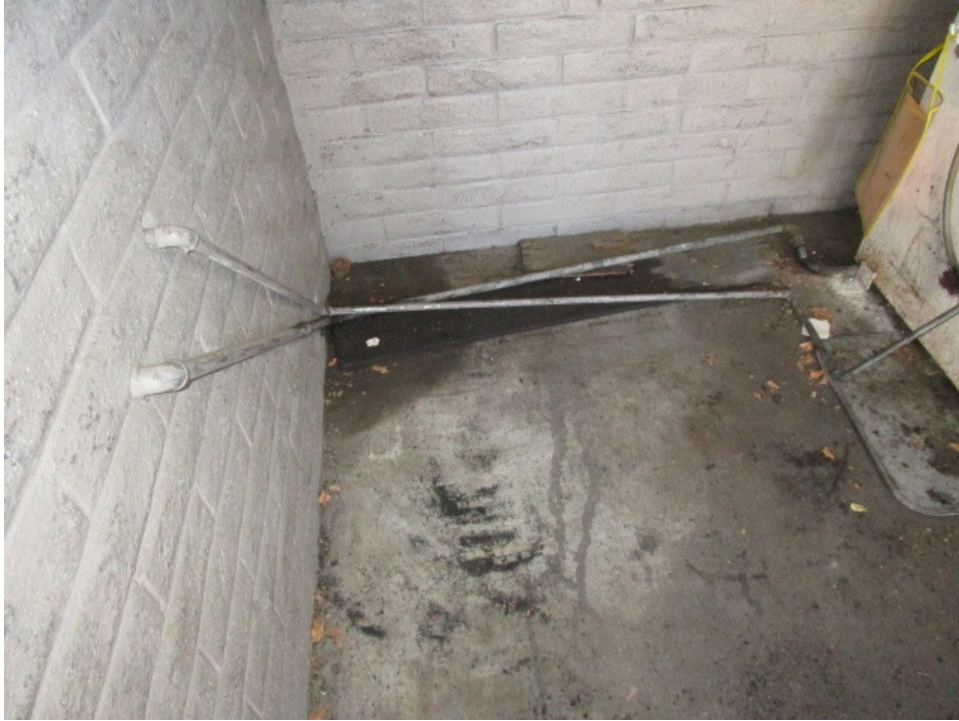
15. Surface staining adjacent to the AST in the enclosure
