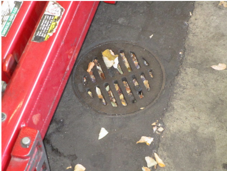
26. Floor drain in the automotive service area
