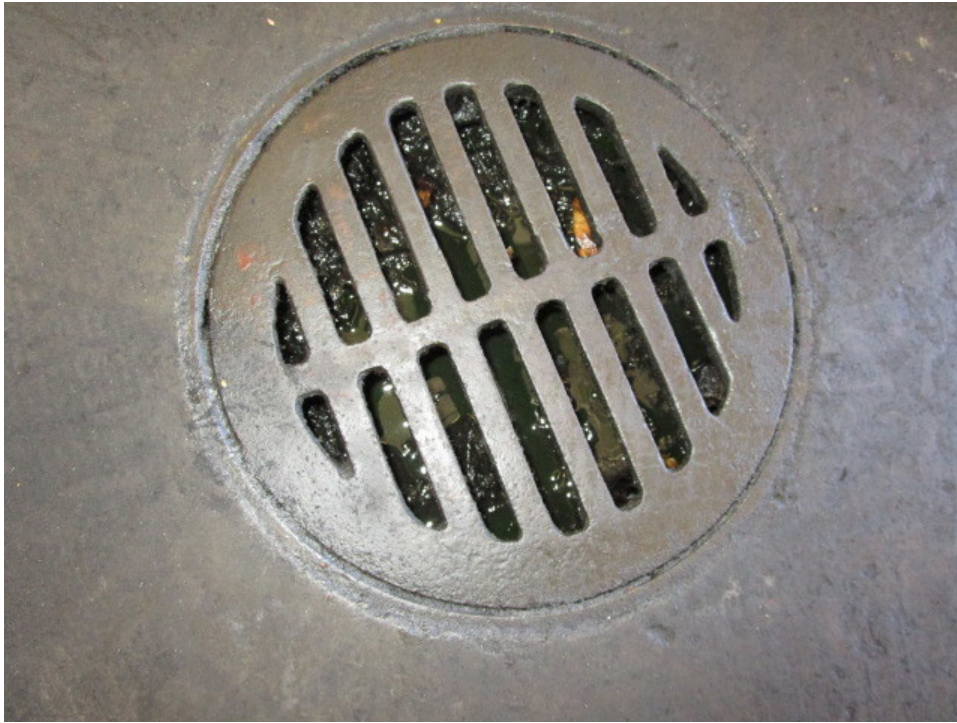
27. Floor drain with oily substance in the automotive service area
