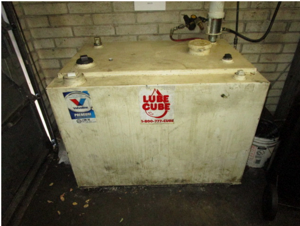
34. New oil AST in the store room
