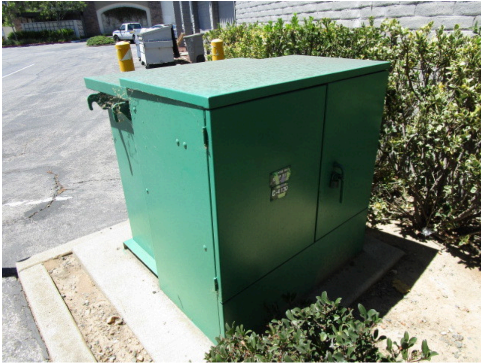
11. Pad-mounted transformer near the southeastern corner of the subject property building
