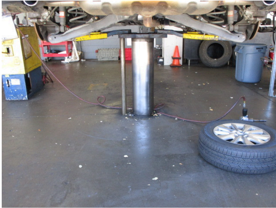
25. Below ground hoist in the automotive service area
