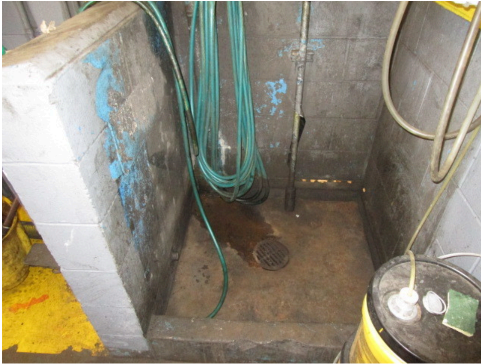
35. Floor sink in the automotive service area
