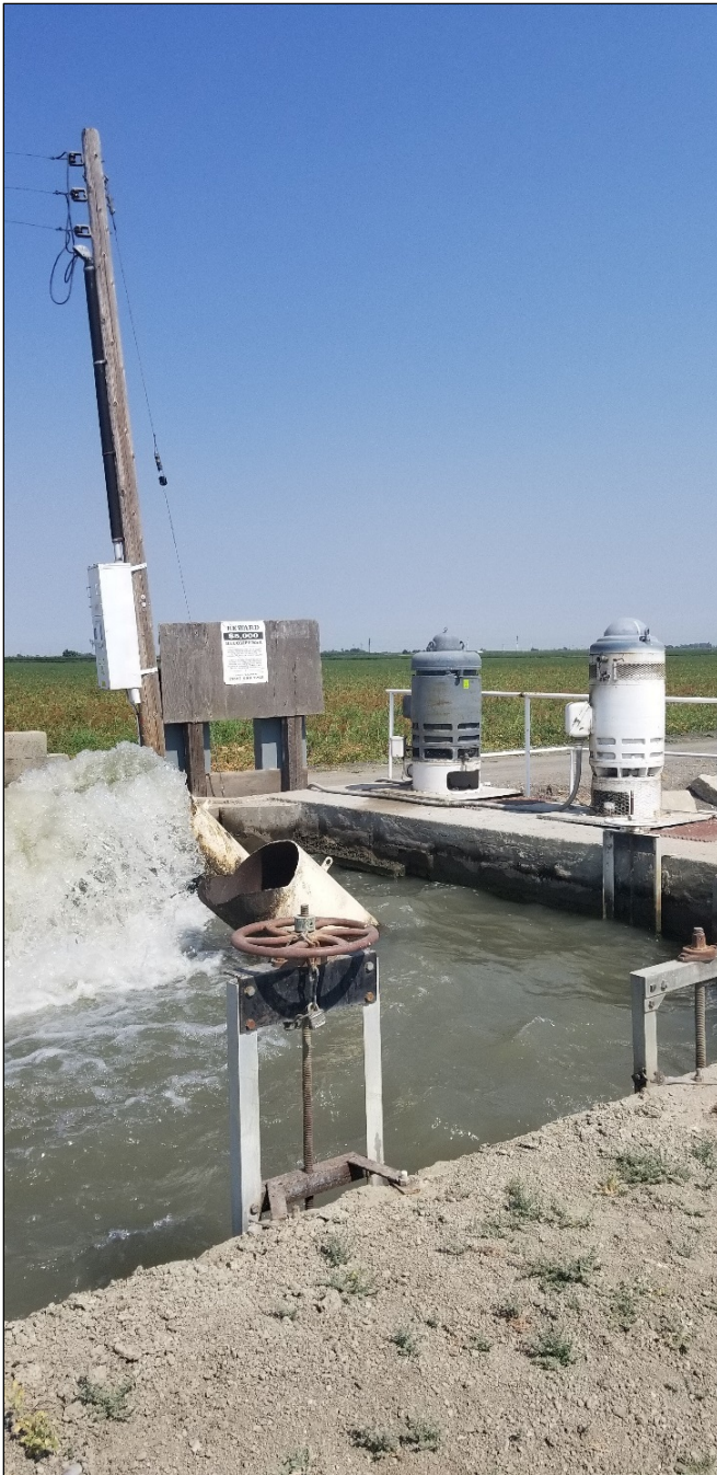
Vertical lift pumps and turnouts, looking west.
