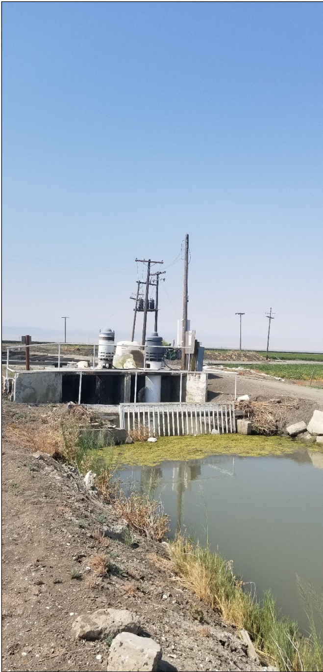
Metal grate debris filter, metal walkway, and vertical lift pump system of TID Slough Canal, looking south.
