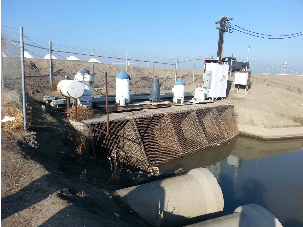
Photo 7: View of off-site Slough Canal lift station pumps at Colorado Road.
