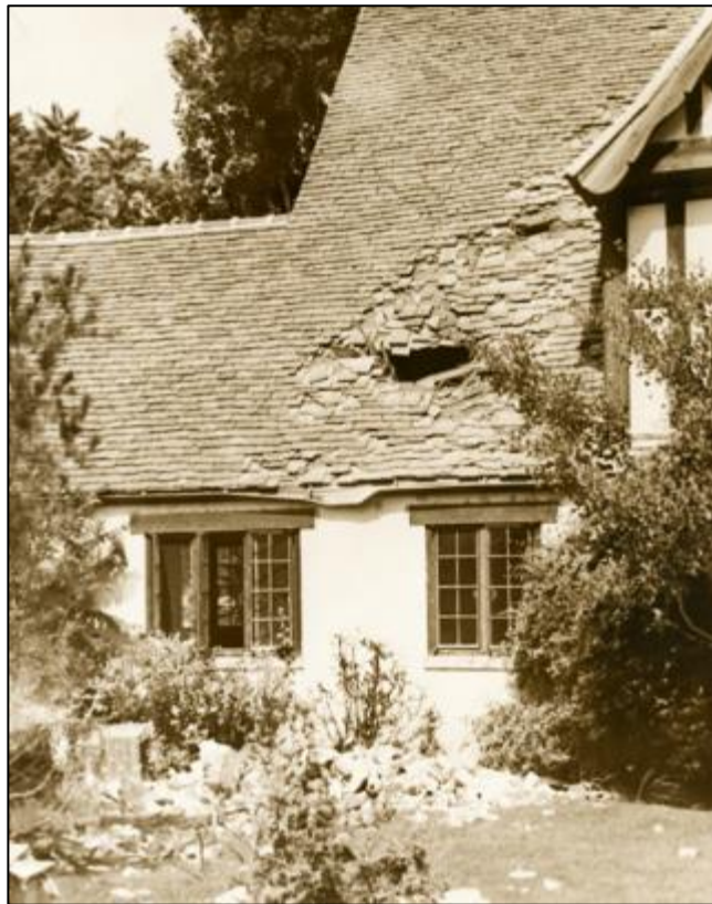
Figure 7. Damage at the CCI (Originally California Institution for Women) from the 1952 earthquake (Chaddock 2015).
