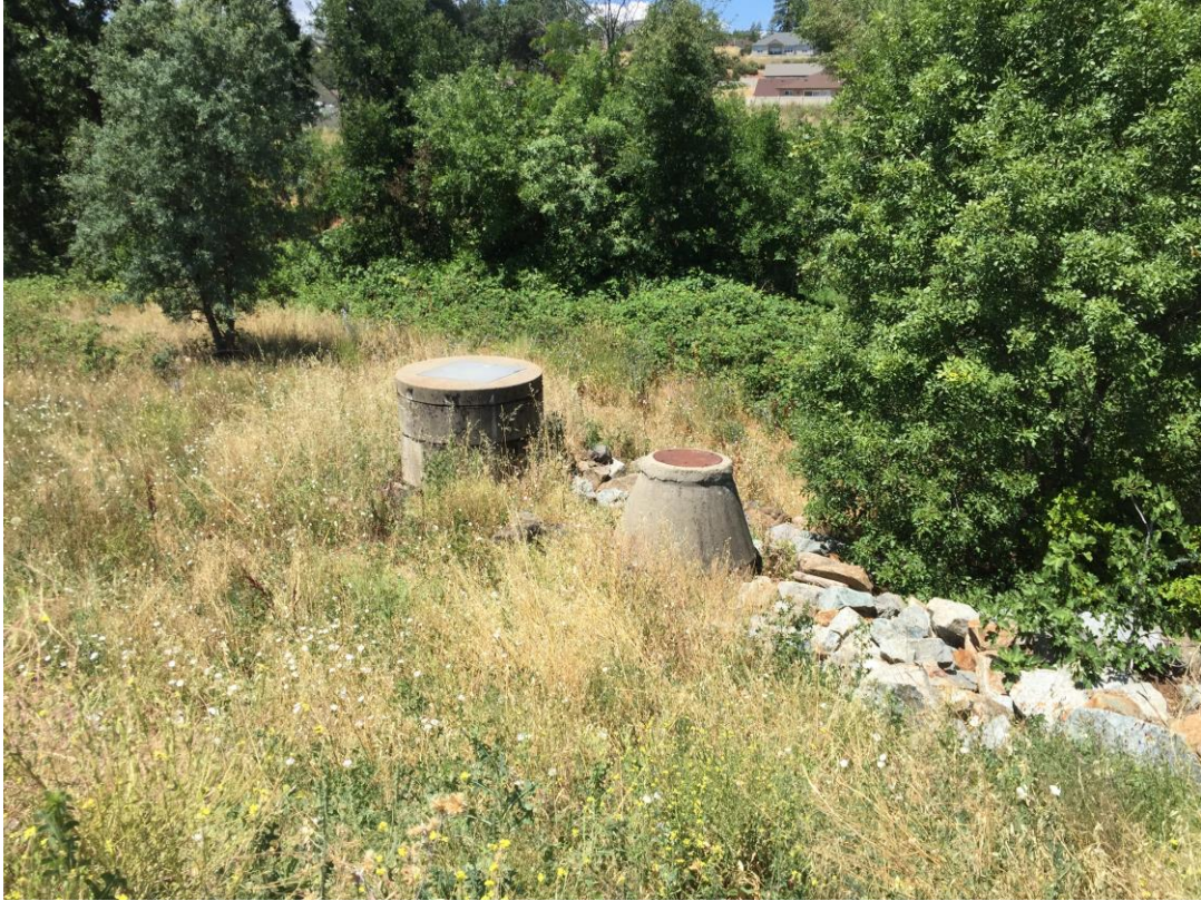
LS 5 diversion and overflow manholes above the Salt Creek riparian zone
