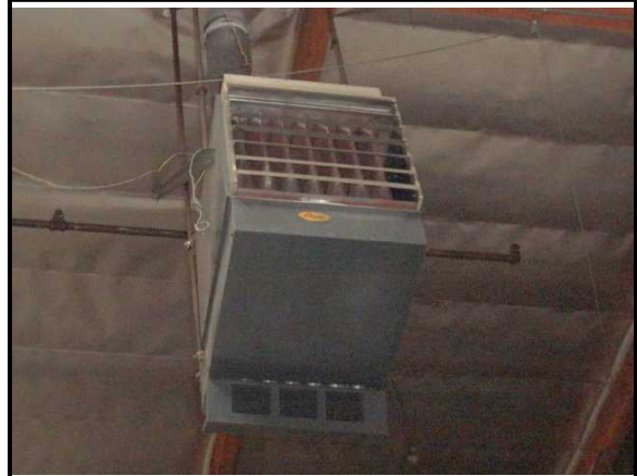
59. Warehouse area suspended unit heater
