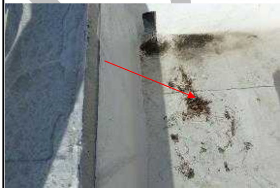
3. Debris on membrane
