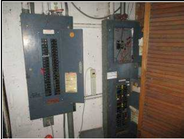
Figure 2.3.3 – Electrical Breaker Panels
