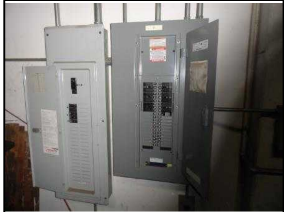
64. Switchgear serving the northeast office area
