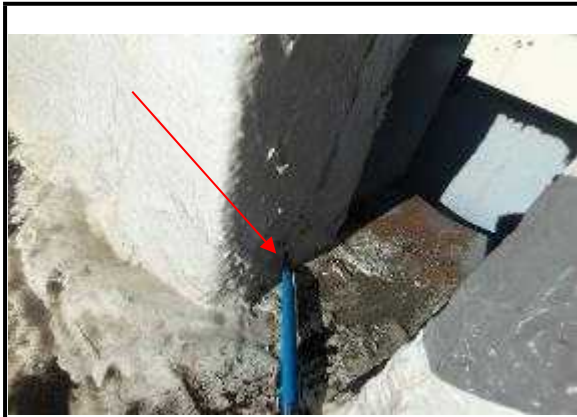
7. Voids in silicone coating
