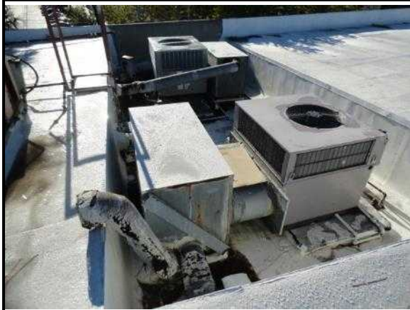
56. Southwest corner office area gas/electric rooftop units
