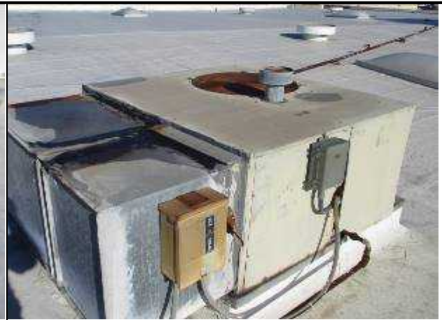
Figure 2.4.2 – Abandoned HVAC unit
