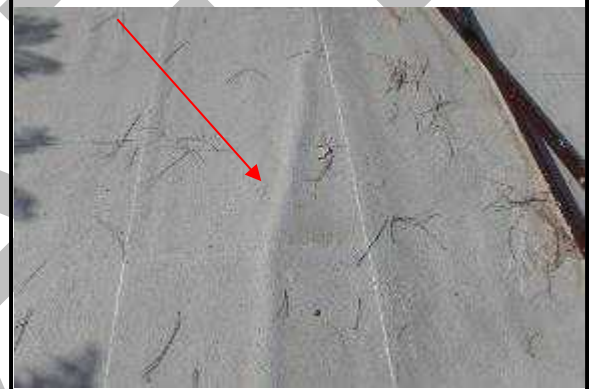
11. Roof membrane ridging
