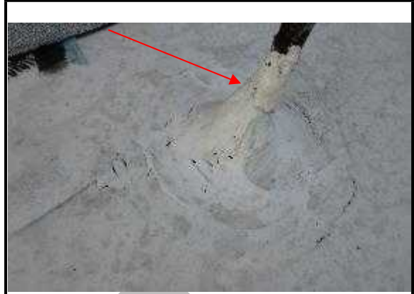
9. Voids in coating at pipe flashing
