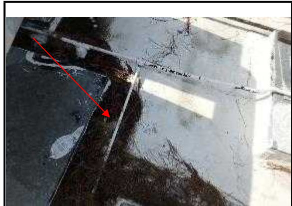
4. Missing support blocking and slip sheet under conduit
