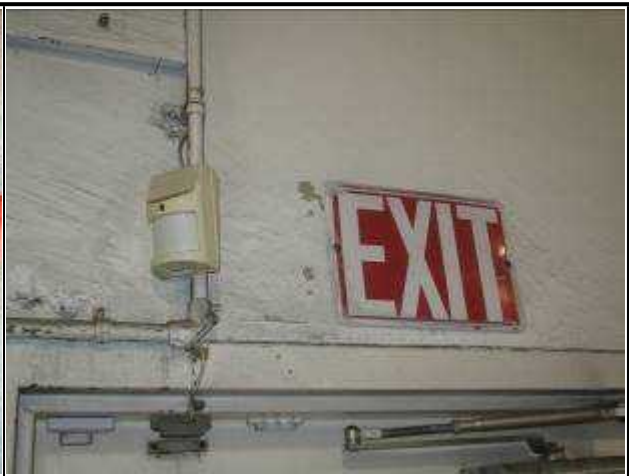
Figure 2.5.4 – Non-illuminated Exit signage
