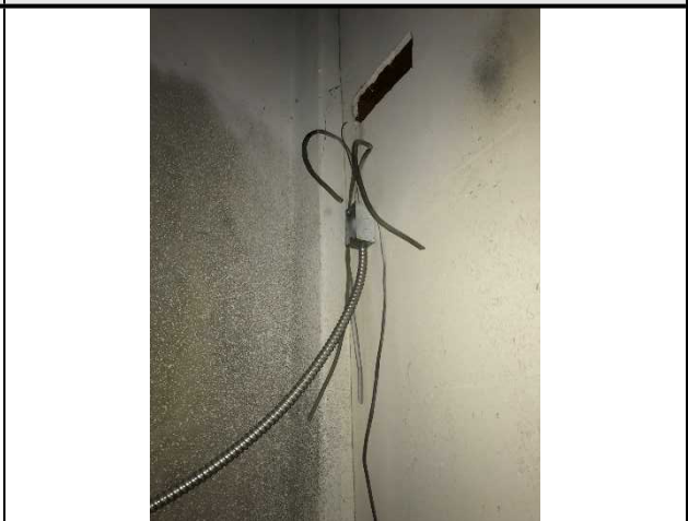
Figure 2.5.6 - Fire sprinkler alarm wiring disconnected
