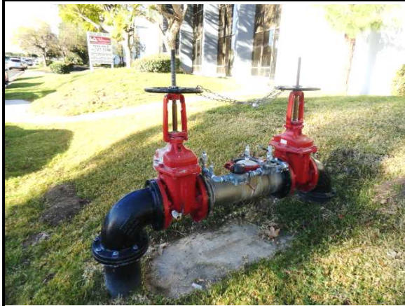
67. Fire sprinkler system detector-check assembly
