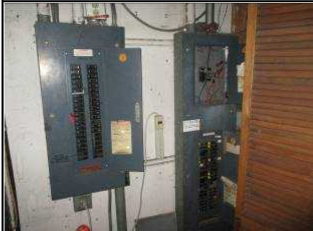
Figure 2.3.3 – Electrical Breaker Panels
