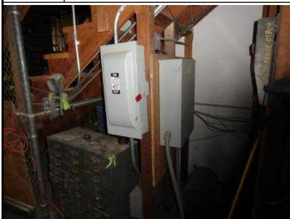
63. Service disconnect serving northeast office area
