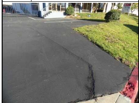
12. Typical asphalt paving condition showing improperly repaired cracks before seal coating
