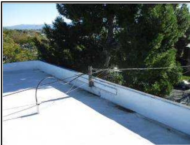
Figure 2.3.1 – Incoming electrical service
