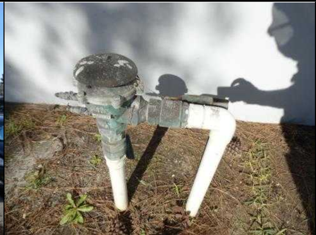
Landscape irrigation system backflow preventer view
