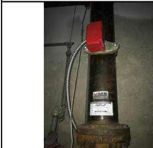
Figure 2.5.5 – Fire sprinkler alarm wiring disconnected
