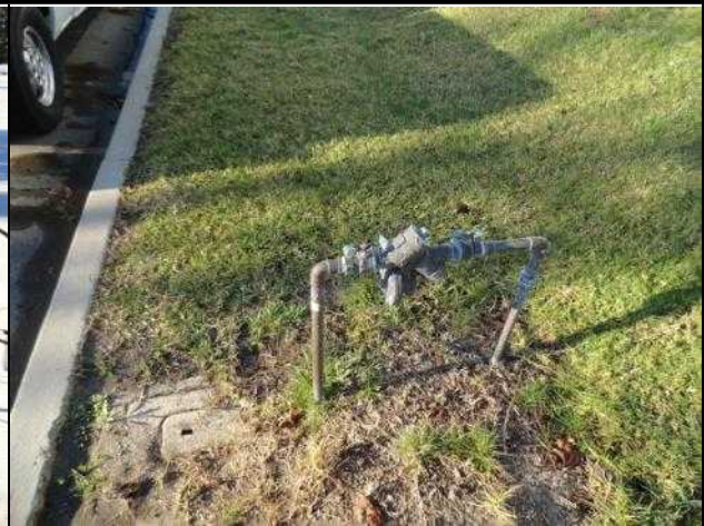
Water meter in yard box with reduced pressure backflow preventer
