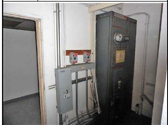
60. General Electric main switchboard, meter and submeters
