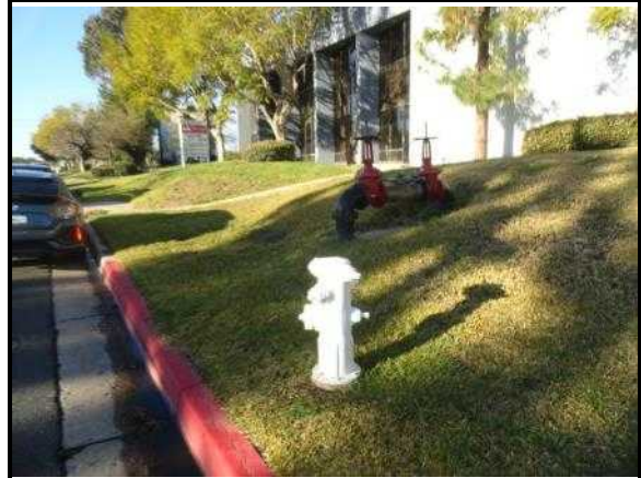
70. Typical fire hydrant
