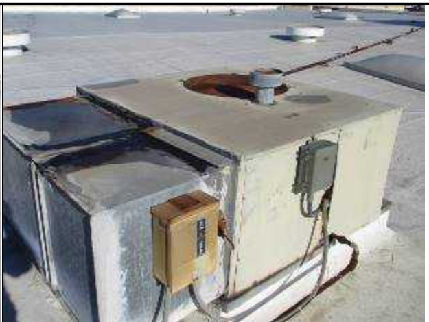
Figure 2.4.2 – Abandoned HVAC unit
