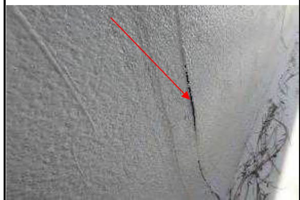
6. Open base flashing seam
