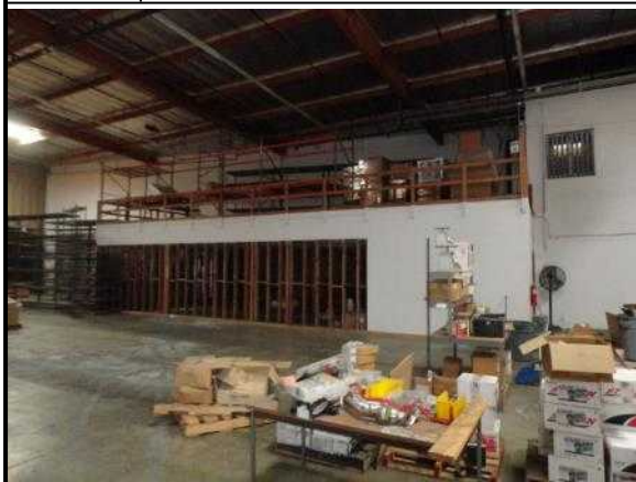
39. Incomplete fire separation wall between warehouse areas and office areas
