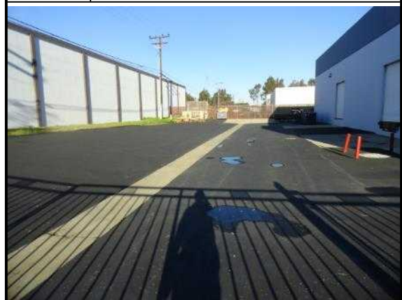
11. Parking spaces were previously striped along the west side of the building but not restriped after sealcoating
