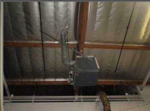
Figure 2.4.4 – Gas Unit Heater
