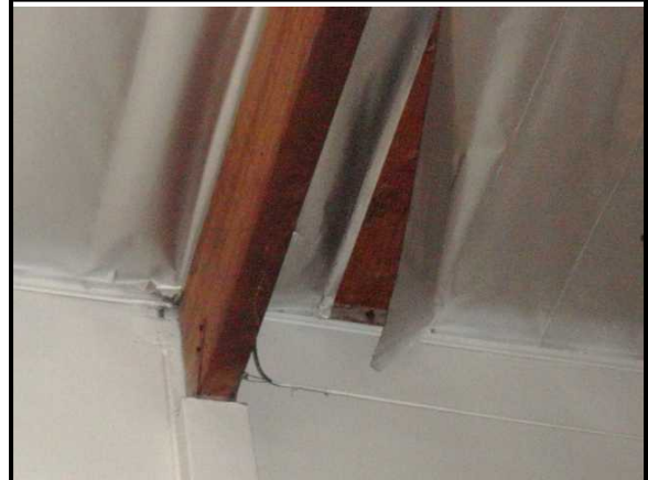
36. Typical structural framing at the exterior wall and pilaster with no seismic hold down bracket upgrading evident
