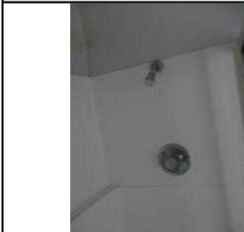
Figure 2.1.5 – Private restroom showerhead
