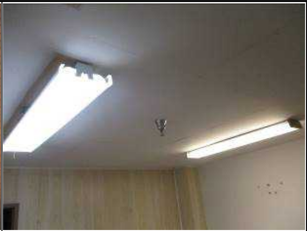
Figure 2.3.4 – Typical T12 fluorescent lighting
