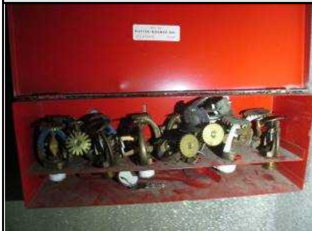
Figure 2.5.3 – Spare sprinkler head box
