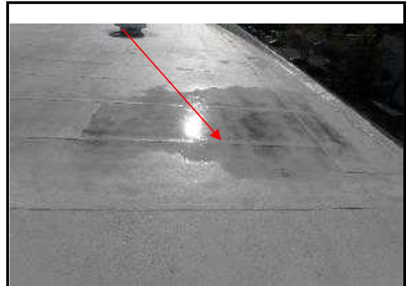
4. Ponding in field
