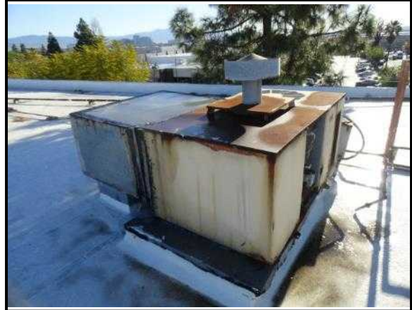
58. Southwest office area gas/electric rooftop unit
