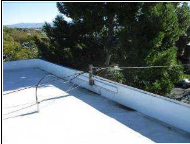
Figure 2.3.1 – Incoming electrical service
