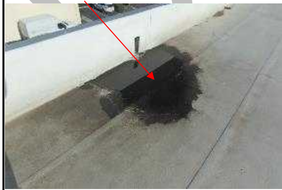
3. Ponding in field
