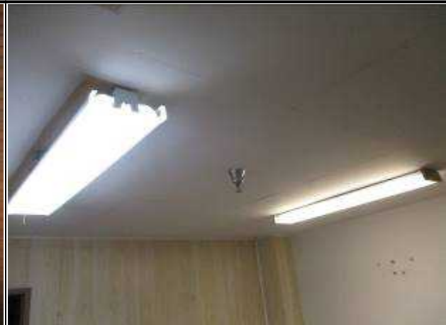
Figure 2.3.4 – Typical T12 fluorescent lighting
