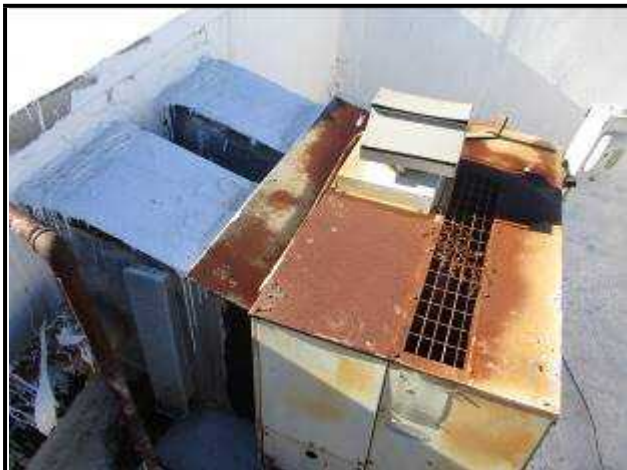
Figure 2.4.1 – Older Day & Night HVAC
