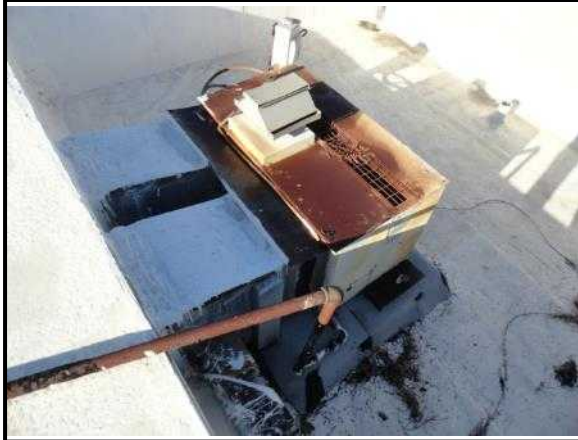
55. Gas/electric rooftop unit serving northeast corner office areas
