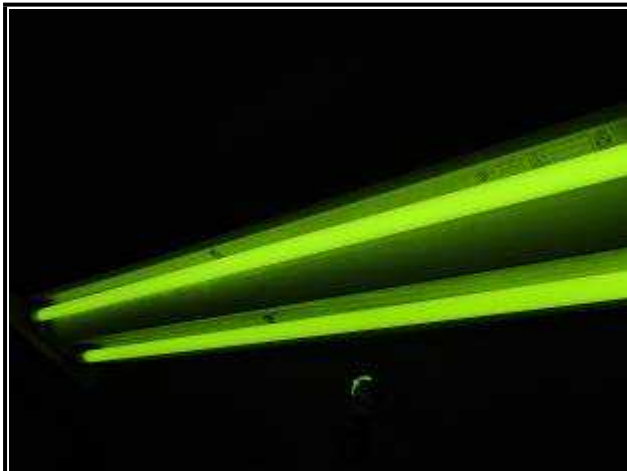
Figure 2.3.5 – Nonfunctional lighting fixtures
