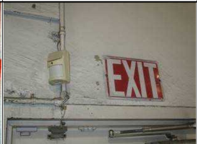
Figure 2.5.4 – Non-illuminated Exit signage
