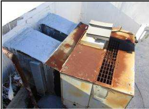
Figure 2.4.1 – Older Day & Night HVAC
