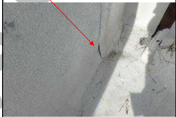
5. Open base flashing seam
