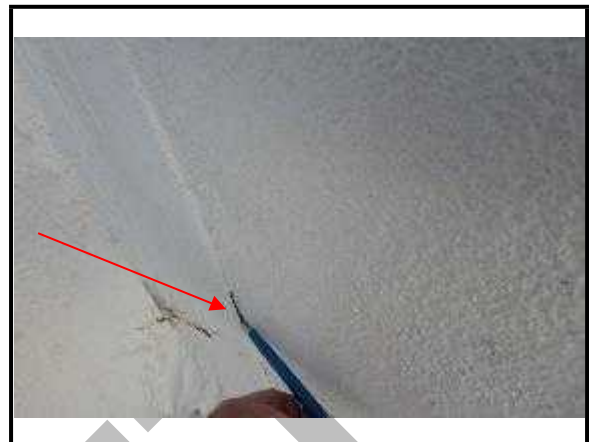
4. Open base flashing seams
