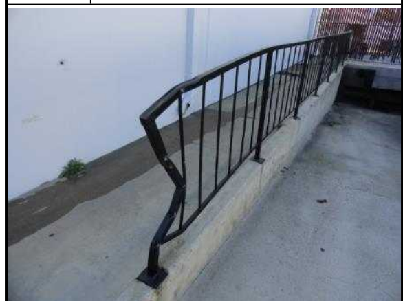
18. Damaged wrought-iron railing at the exterior loading dock
