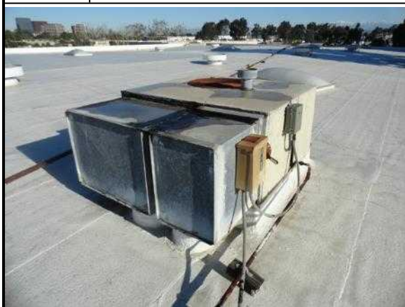
57. Southwest office area gas/electric rooftop unit
