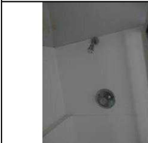
Figure 2.1.5 – Private restroom showerhead
