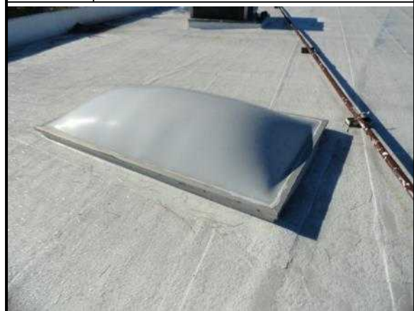
29. Typical skylight has no fall protection
