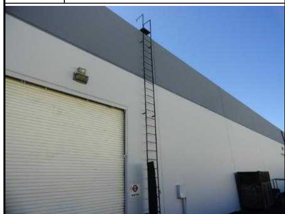
30. Roof access ladder does not have a safety cage or proper security shield to control access
