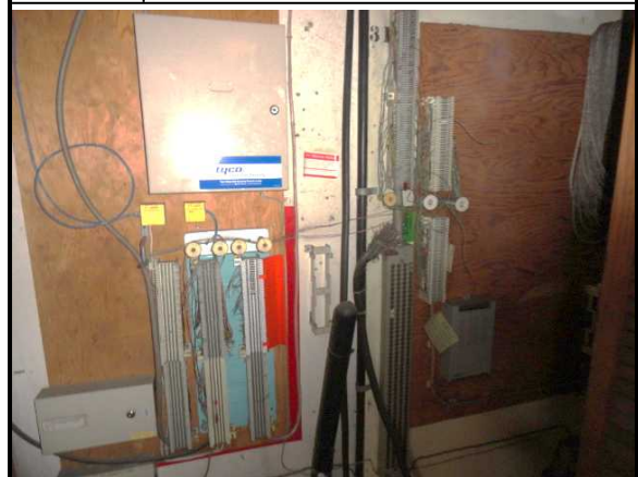
71. Security monitoring panel
