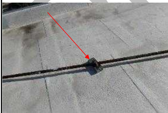
9. Blocking lacks slip sheet
