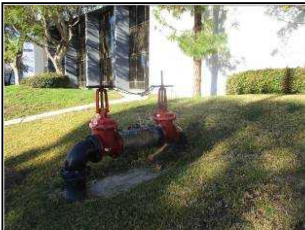
Figure 2.2.1 – Fire sprinkler water piping
