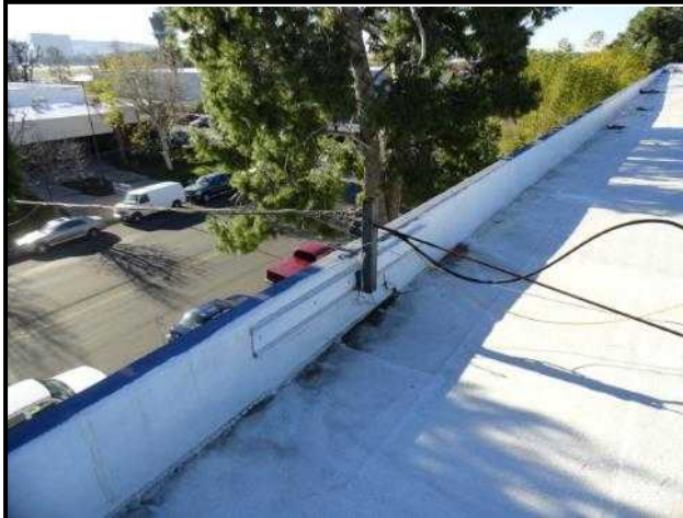
Power for the sub-tenant space at the northeast corner of the building is provided overhead down to electrical panel and main breaker
