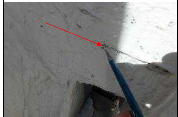
6. Exposed webbing at scupper
