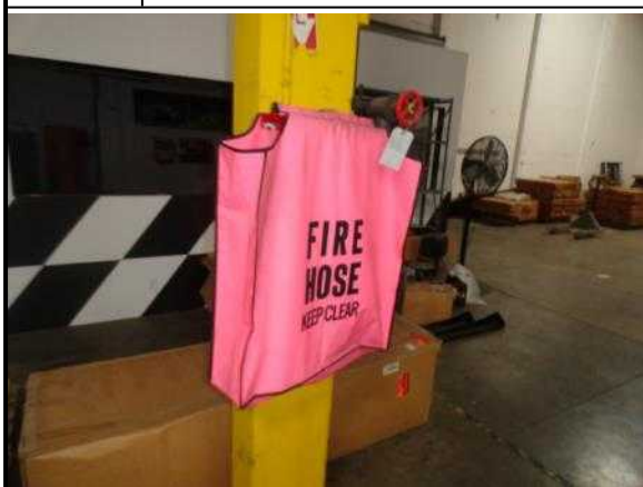
69. Fire hose drop in warehouse area
