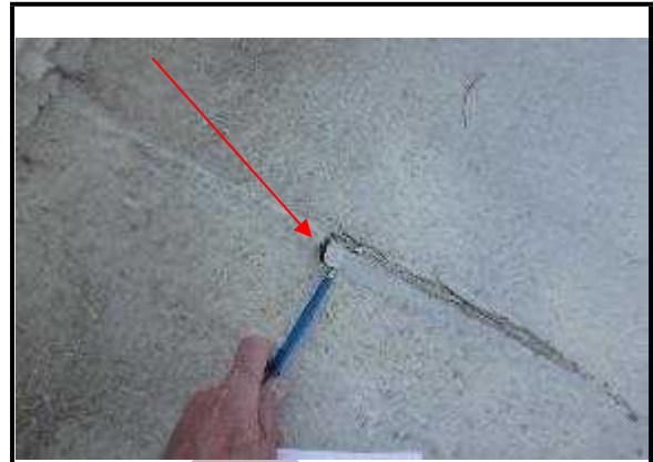
10. Peeling coating at field lap
