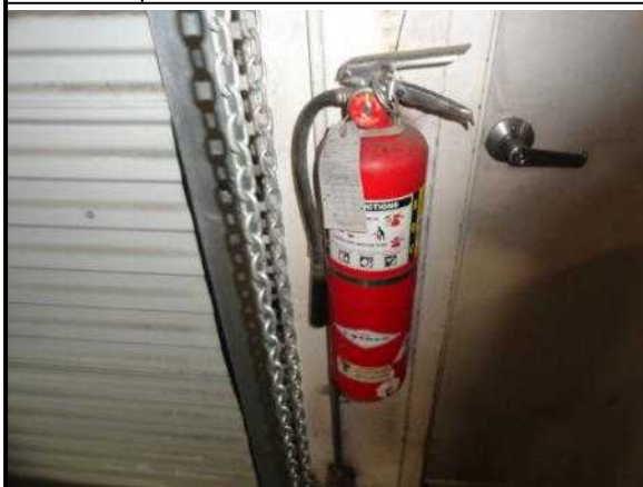
68. Typical portable fire extinguisher
