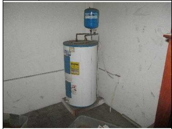
12. Hot water heater in north west office portion. Note no seismic straps.
