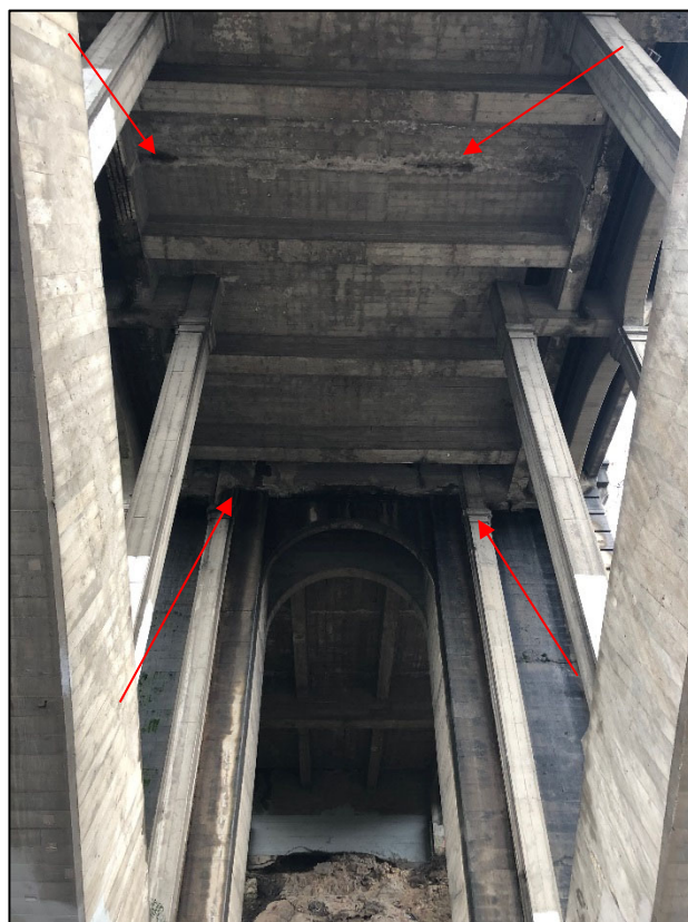
Image showing cracking and spalling (with exposed rebar) on the Holly Street Bridge. Source: GPA Consulting (2019).
