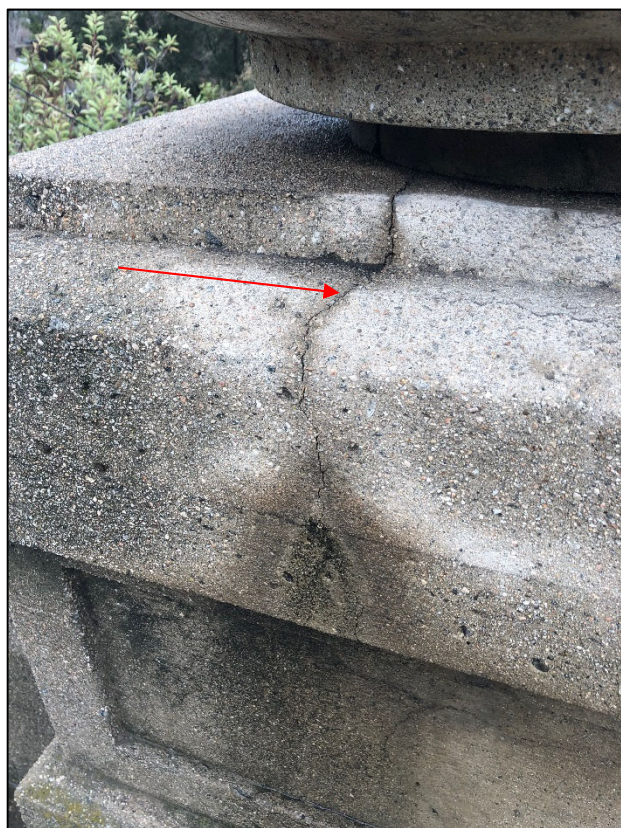
Image showing typical cracking on the Holly Street Bridge. Source: GPA Consulting (2019).
