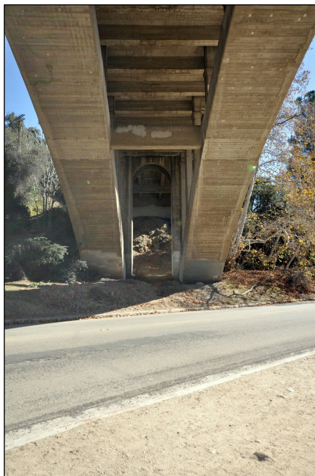
The Holly Street Bridge arch from below the bridge, view facing southeast. Source: GPA Consulting (2018).
