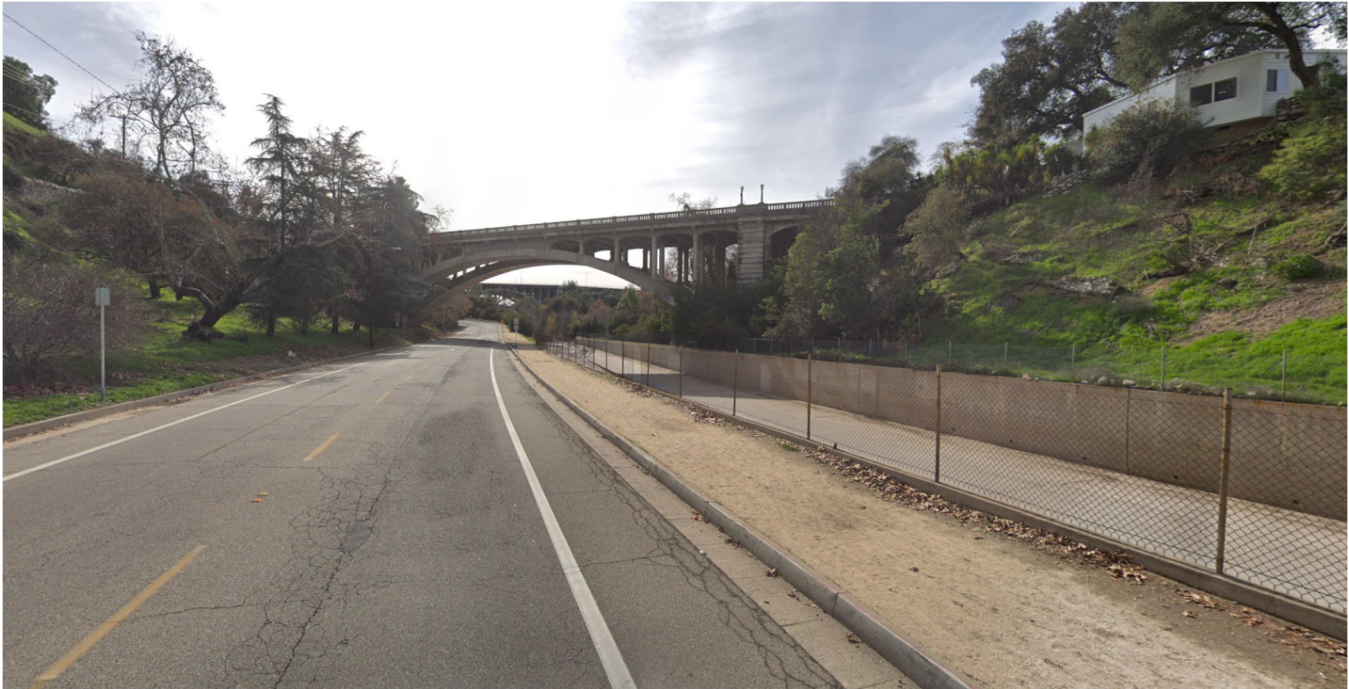
Image showing a view of the existing Holly Street Bridge and North Arroyo Boulevard, looking south towards the bridge.
