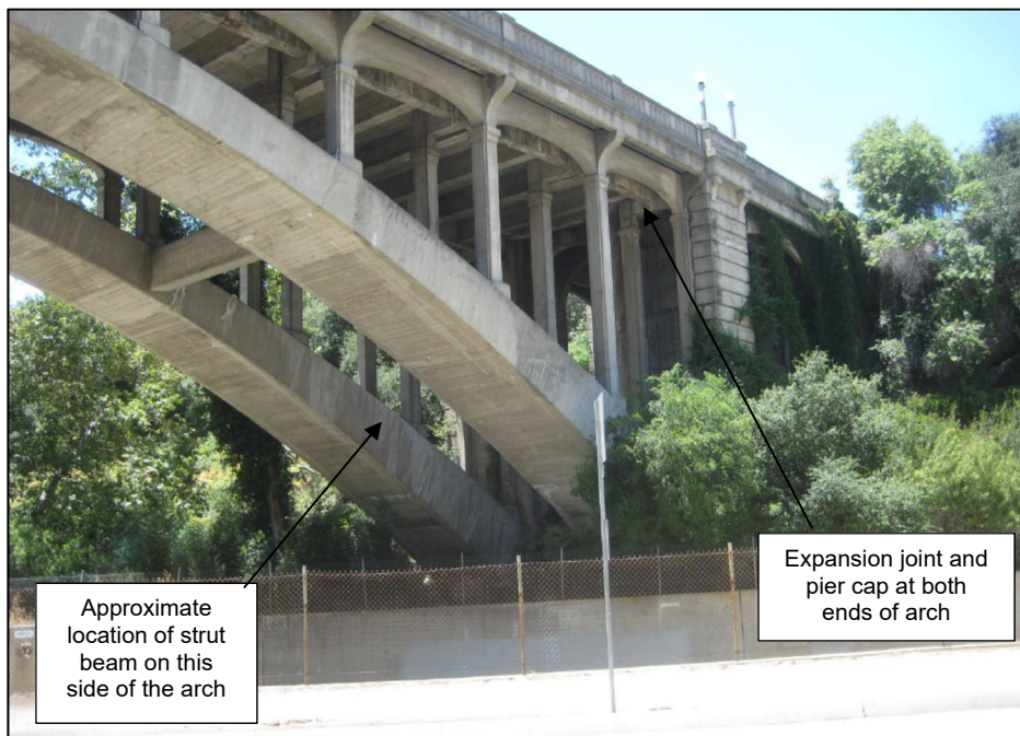
Annotated view of the bridge showing locations of proposed work, view facing west. Source: Dokken Engineering (2018).
