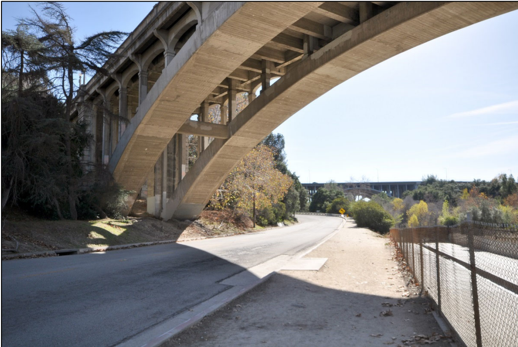
The Holly Street Bridge arch, struts, spandrel columns, view facing south. Source: GPA Consulting (2018).
