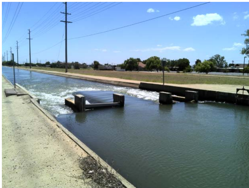
Photo 753. Feature B - metal box (left) on the eastern berm of the canal, associated with the dam. Facing southwest.
