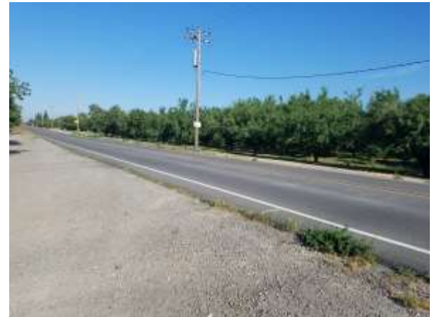
Photograph 6. View of pole-mounted transformer west of the canal bridge along E Keyes Rd, looking northwest.
