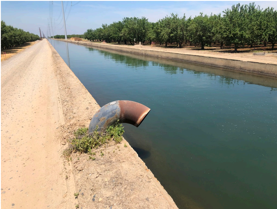
Photograph 2. Open pipe along Ceres Main Canal with sparse ruderal vegetation shown. View to the north.
