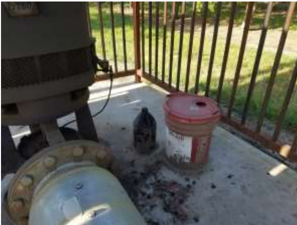
Photograph 4. View of lubricant containers for water pump.
