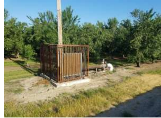
Photograph 3. View of the water pump north of the canal bridge, facing northwest.
