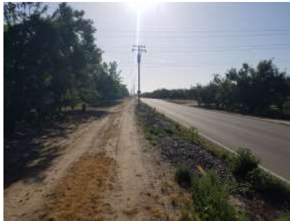
Photograph 11. View of pole-mounted transformer east of the project site, facing east.
