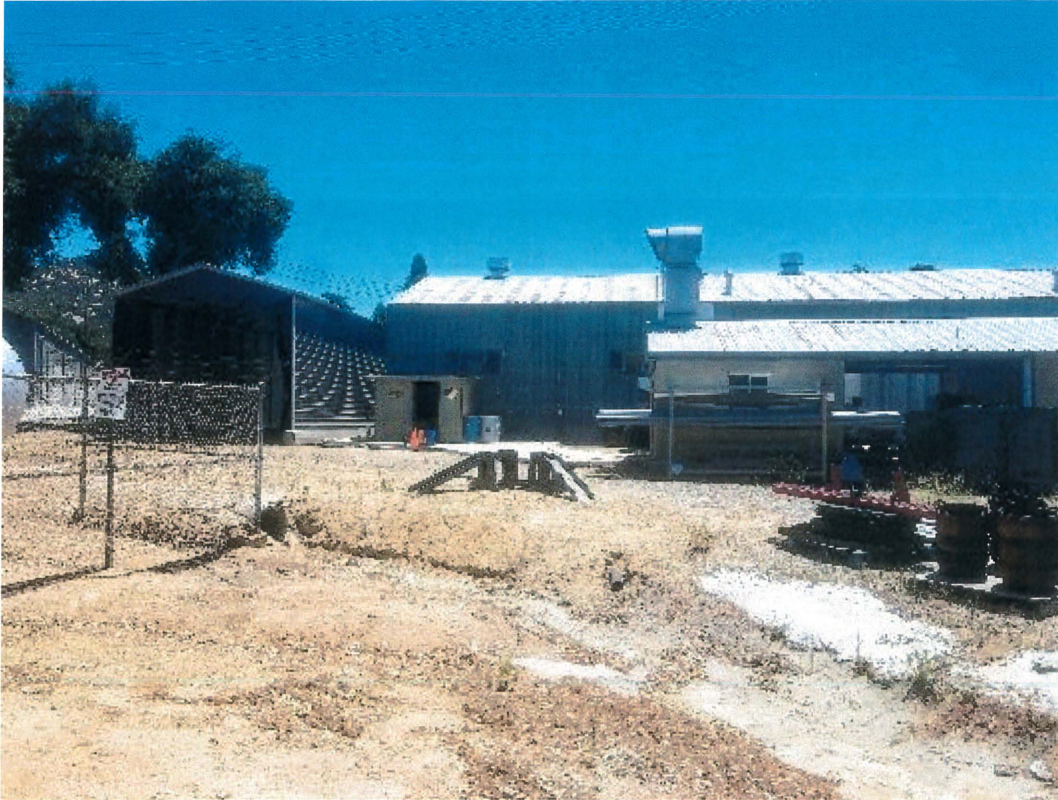
Photo 3: Looking East, trench run from project site to electrical panel on Mechanics Building.
