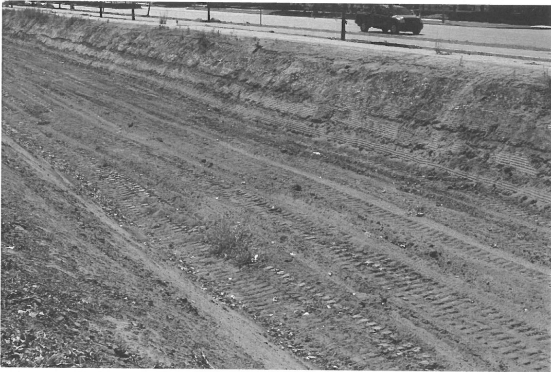
FIGURE 2 : TYPICAL CREEK CONDITIONS AFTER REGULAR MAINTENANCE. VIEW CLOSE TO PROPOSED BRIDGE CROSSING. (PHOTO TAKEN JULY 23, 2016)
