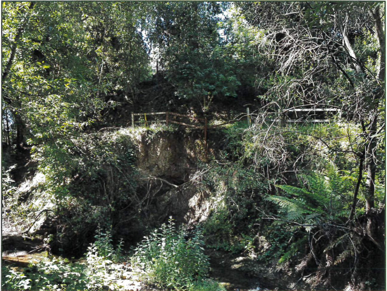
Figure 4. The washout area upstream of the project area that closed a segment of the Center Trail, requiring the proposed Center Bridge project to reopen the trail.
