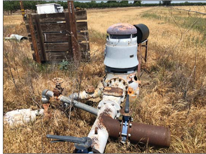
PHOTOGRAPH 13: View of motor and electric engine
