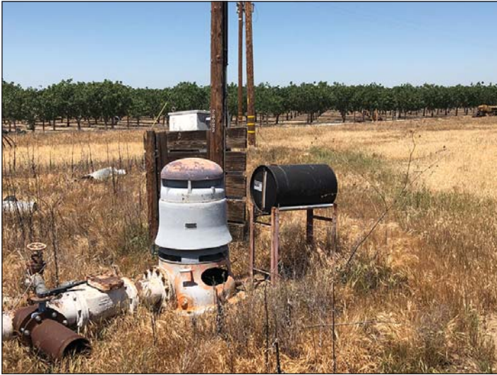
PHOTOGRAPH 12: View of 30-gallon AST
