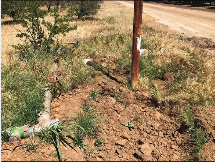
PHOTOGRAPH 1: Disconnected subterranean pipes
