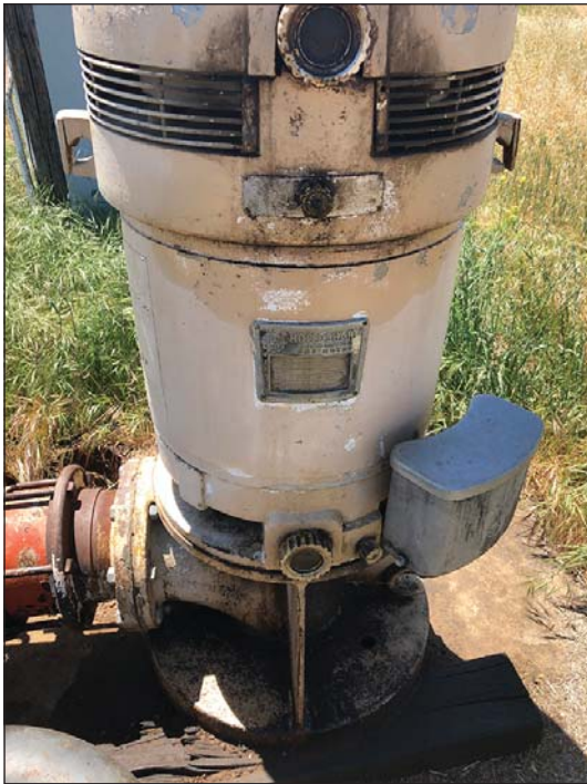
PHOTOGRAPH 4: View of electrical motor
