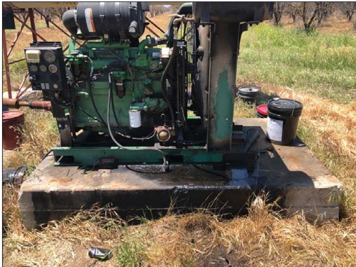
PHOTOGRAPH 10: Diesel Motor and leakage
