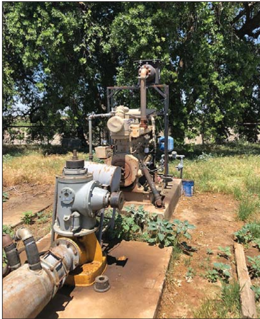
PHOTOGRAPH 15: View of motor and electric pumping system
