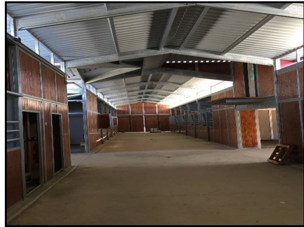
Photograph 8. View of interior of horse stable with enclosed metal stables with wood panels. The interior is protected with a commercial, automatic fire sprinkler system.
