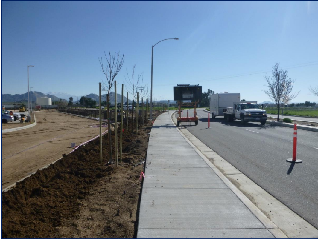
Figure 5-5 View of commercial developments adjacent (north) to Perry Street and Indian Avenue, view to the southeast.
