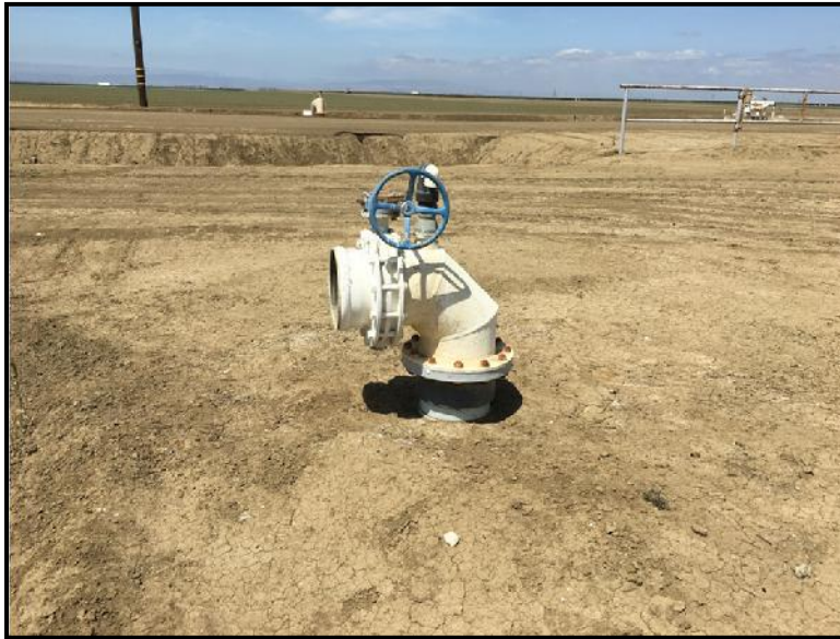
Example of irrigation piping located throughout Site
