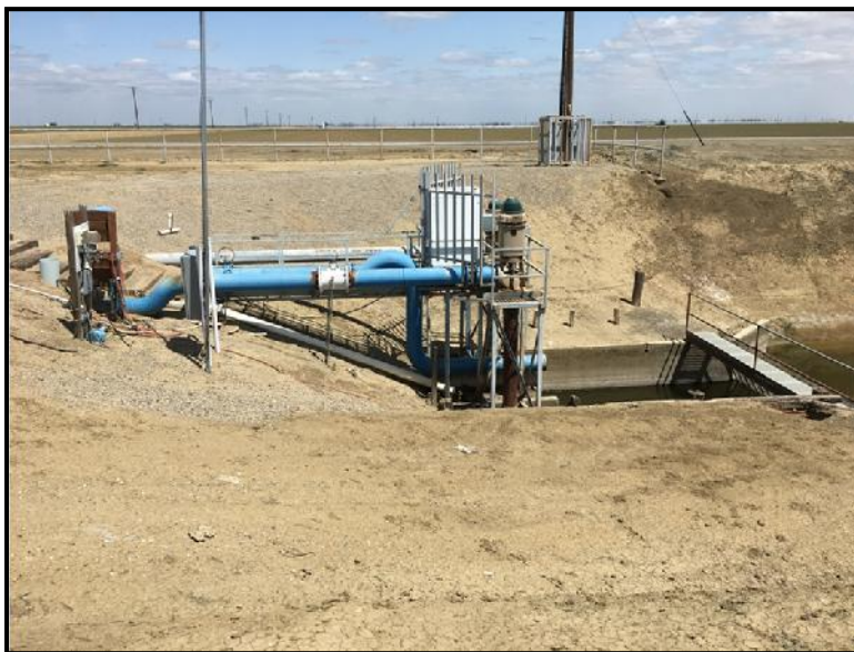
Well-head, pump, and irrigation equipment in northwest corner of Site
