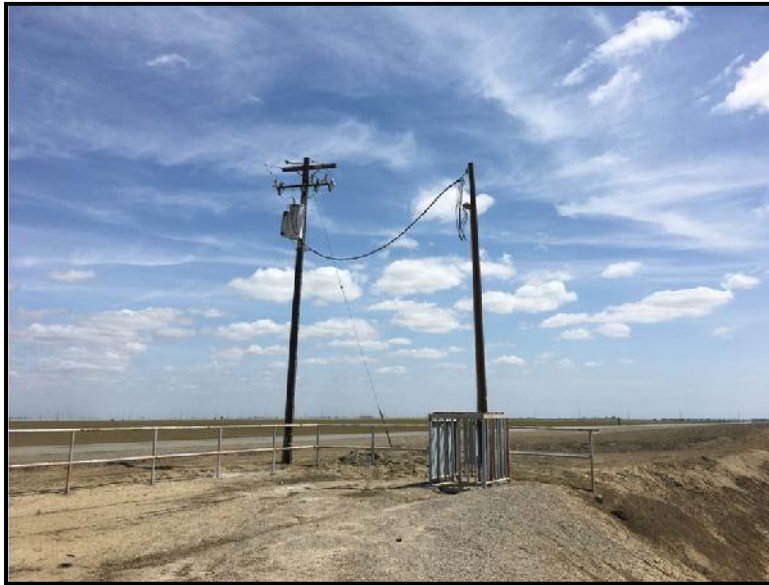
Pole-mounted transformer located on Site
