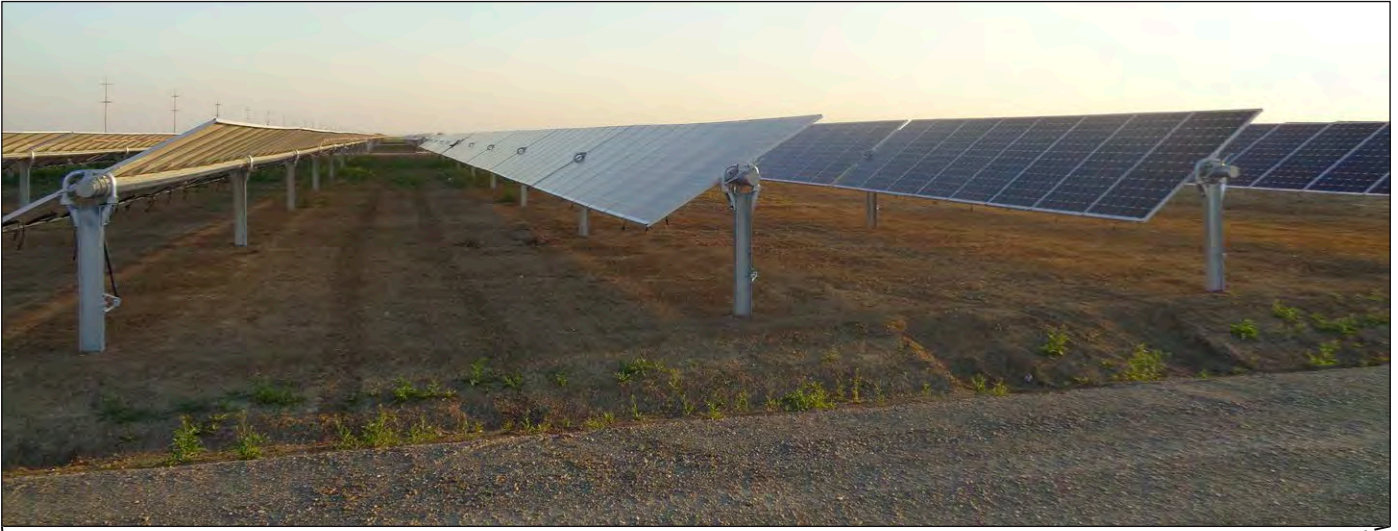
Solar PV Modules on Horizontal Trackers
