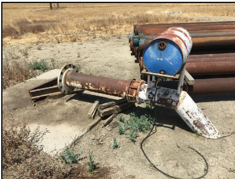
Well with associated hydraulic tank in northeast corner of Site
