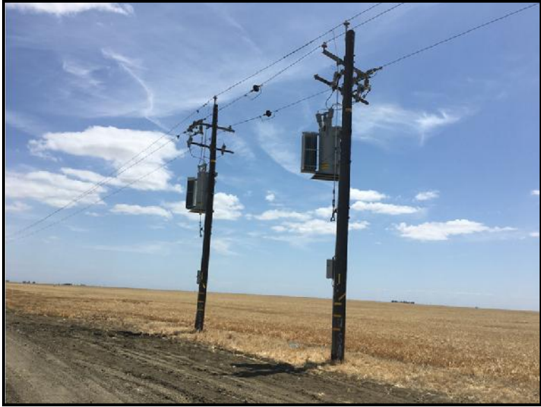
Pole-mounted transformers on Site
