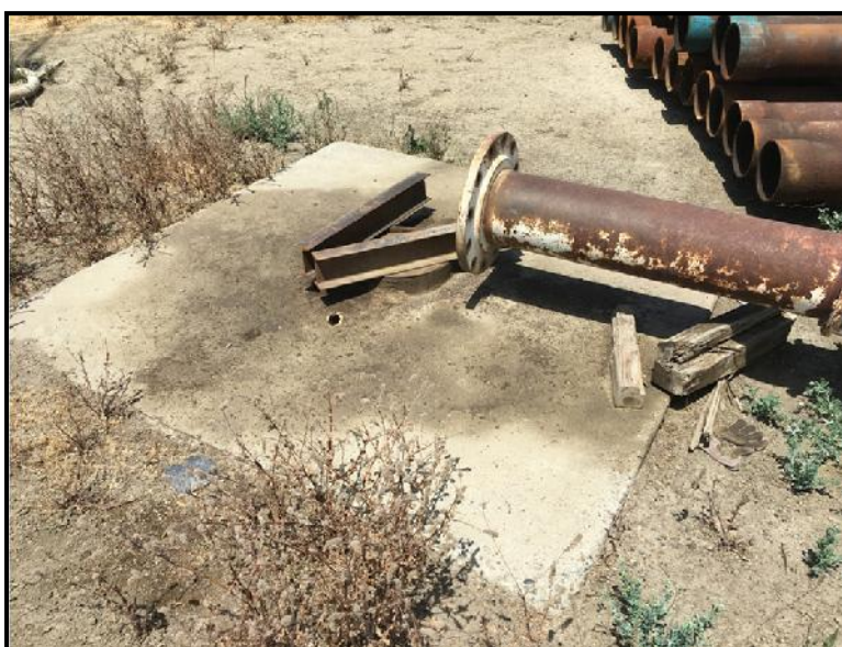
Stained concrete at well in northeast corner of Site
