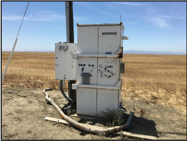
Electrical utilities in northeast corner of Site
