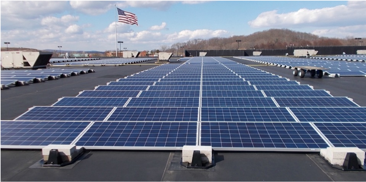
Typical Roof Mounted “Self-Ballasted” Solar System
