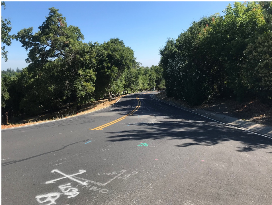
6. View of Taaffe Road looking east (downhill) from lower Dezahara Way intersection
