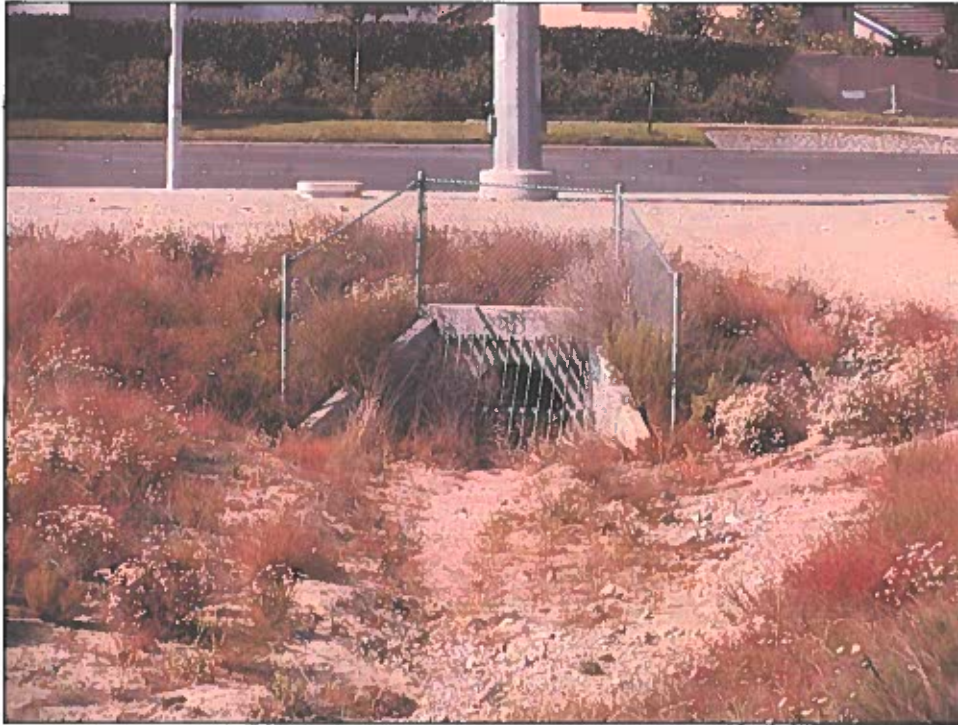
PHOTOGRAPH 7: View of drainage feature and culvert on project site as seen facing Base Line Road (southwest corner).
