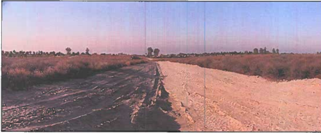
PHOTOGRAPH 1: View of earthen drainage feature as seen from north boundary facing south.
