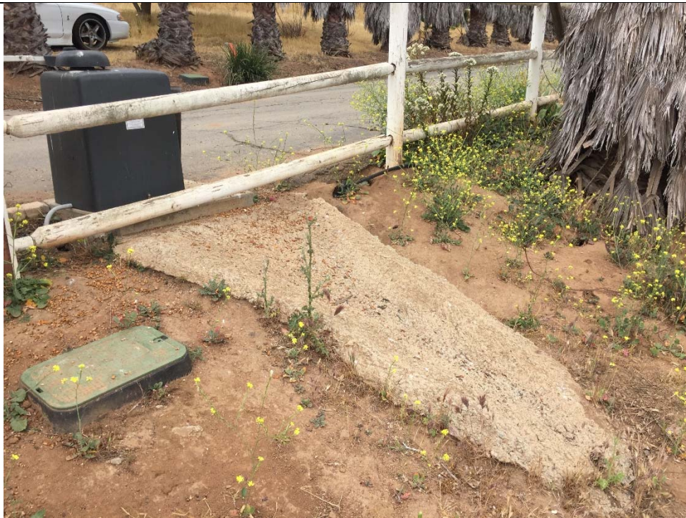
Photo 6: Six foot long concrete v-ditch located at the middle of the southern boundary, facing south.
