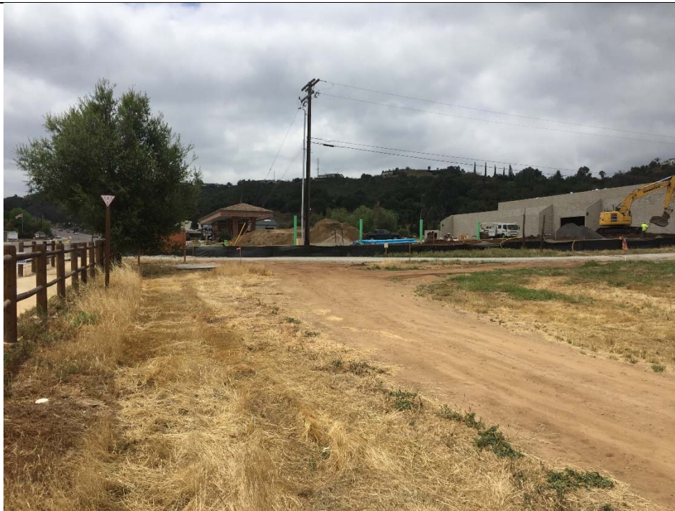
Photo 4: Southeastern corner of site, active construction occurring within southern 100-foot buffer behind black silt fence, facing south.
