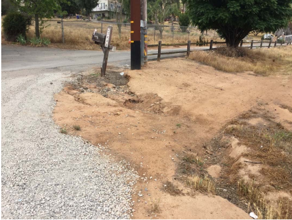
Photo 7: Erosional rill starting at mailbox, approximately 100 feet in length before turning into sheet flow, west of unnamed gravel, facing south.
