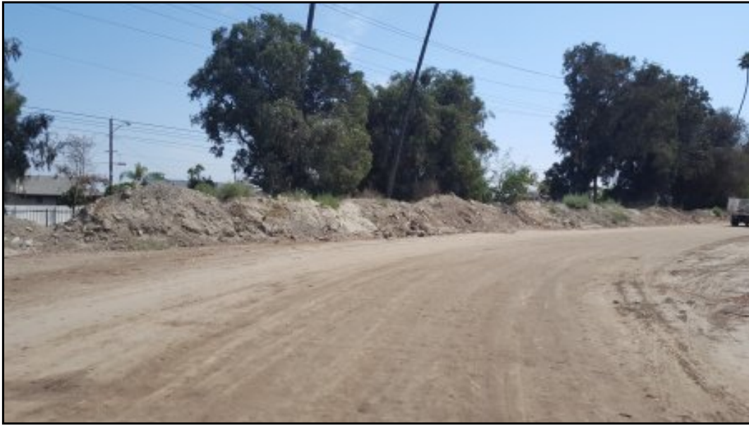
7 : View of stockpiled soil material near northern portion of site adjoining West Cerritos Avenue generated from site grading.
