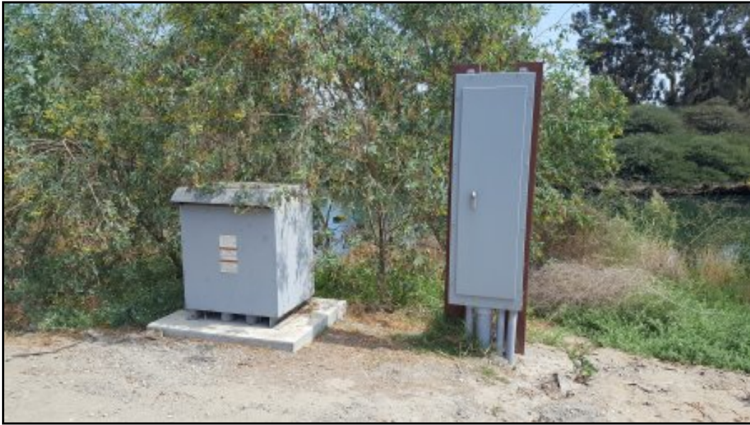
9 : View of pad-mounted transformer located south of the pond in central portion of site.
