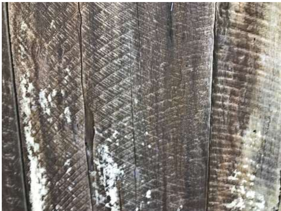
Photo 7: Board showing sawmill marks.
