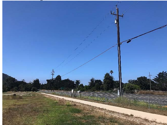
Photograph 4. Aerial Installation: Looking south along SR 1 just south of Rio Road intersection.
