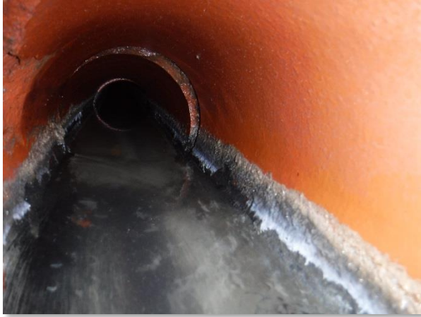
Southeast Monitored Influent Pipe – 2336 Monroe St
