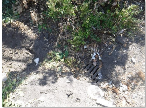
Uncovered storm drain grate near original proposed sanitary sewer manhole – 2330 Monroe St
