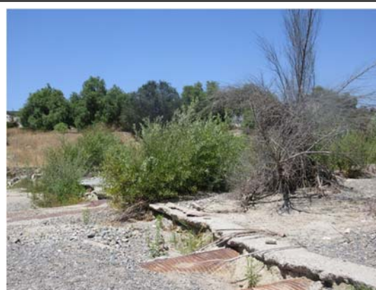
Removal of the Arizona crossing would require excavation of approximately 700 cy of concrete, riprap, and rubble, resulting in temporary construction noise within a recreational land use area.
