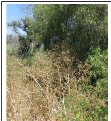
Cracks in the unstable fill added to the streambank have allowed the growth of non-native species adjacent to the riparian vegetation along San Juan Creek.
