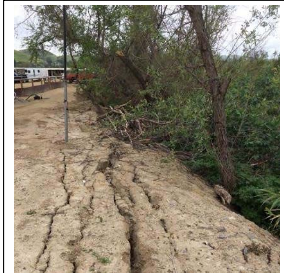
The fill material associated with the 2011 emergency repairs is currently unstable and shows signs of cracking and sloughing due to poor compaction at the time of placement.
