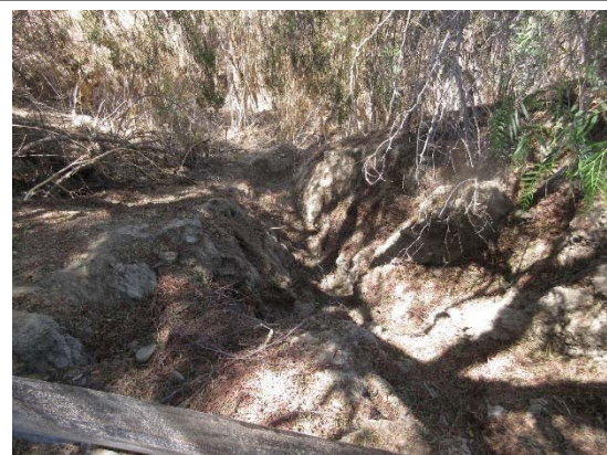
The proposed Project would remove poorly compacted soil to replace with native soils and install rip-rap and other streambank stabilization measures to maintain the creek's eastern embankment.
