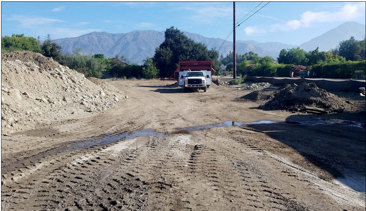
Figure 4. Overview of the project area. (Photograph taken on July 29, 2019; view to the north)
