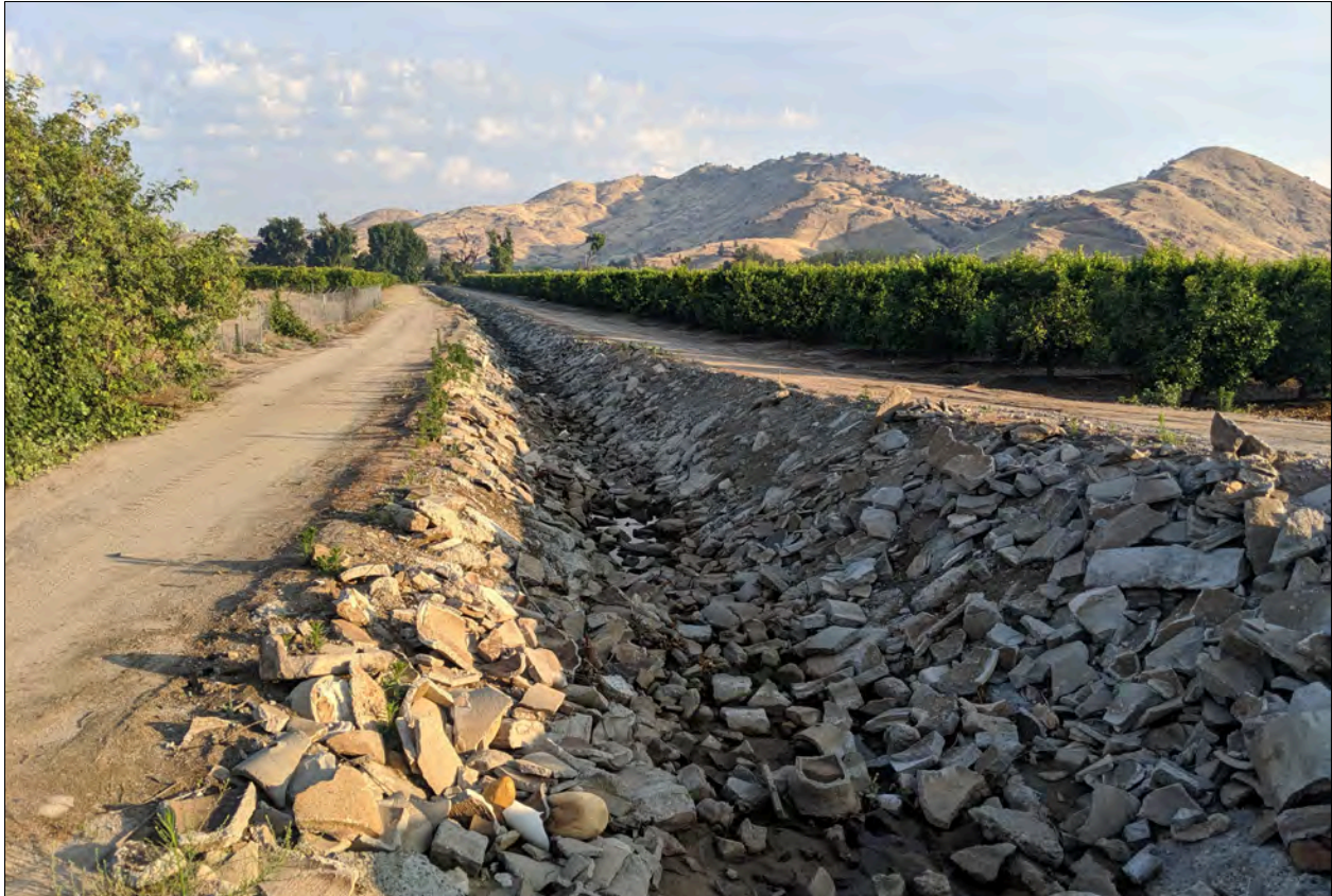
Figure 8. Photograph showing a concrete riprap-lined irrigation canal 20 feet east of the Project site.
