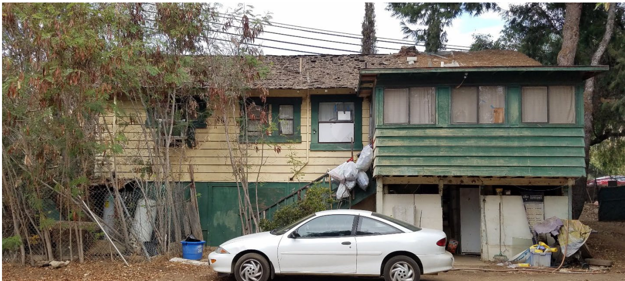
Figure 1. South façade, showing the original residence with the 1953-64 addition (right), facing north (3629-25, 11/19/2019).
