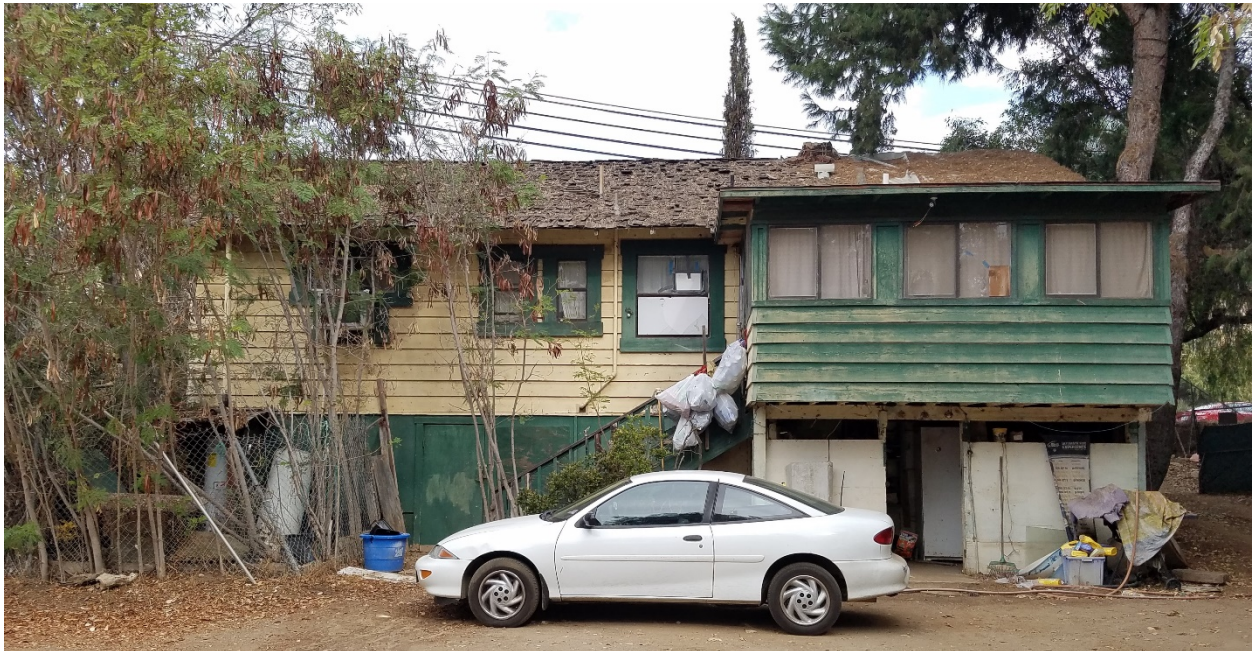
Figure 13. 3629 Willow Glen Drive (P-37-039117) South Façade, showing the 1953-64 addition (right), facing north (3629-25, 11/19/2019)
