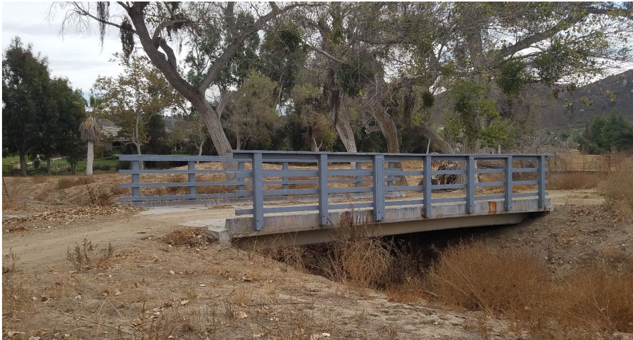
Figure 7. Modern golf cart bridge on The Lakes Golf Course, facing SE (LA-03, 11/19/2019)
